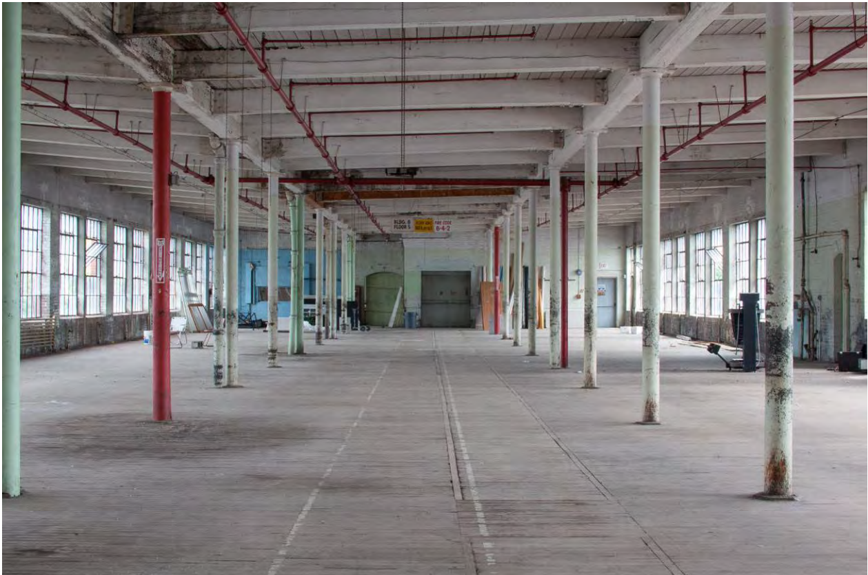
Photo 49. 5 th floor of Building H looking north; the structure changes from steel frame to timber at the roof. Steel rails installed in the floors eased the job of moving boots and shoes on racks from the making rooms on the upper levels of the manufacturing building to the pressurized vulcanizer chambers on the second floor of Building K.
