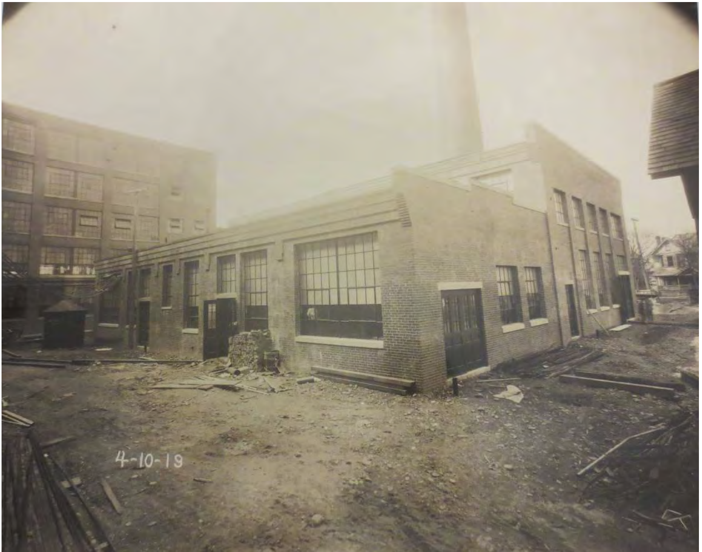
04-10-1919 Construction Photo of Building M, New Boiler House and Chimney; Lycoming Rubber Company; looking southwest; Lockwood Greene Records, Archives Center, National Museum of American History, Smithsonian Institution
