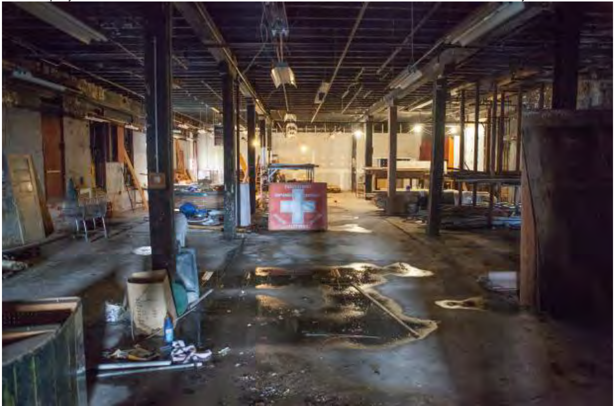
Photo 12. View of ground floor of Building A looking east toward wood frame demising wall separating the community woodshop from the remainder of the space.
