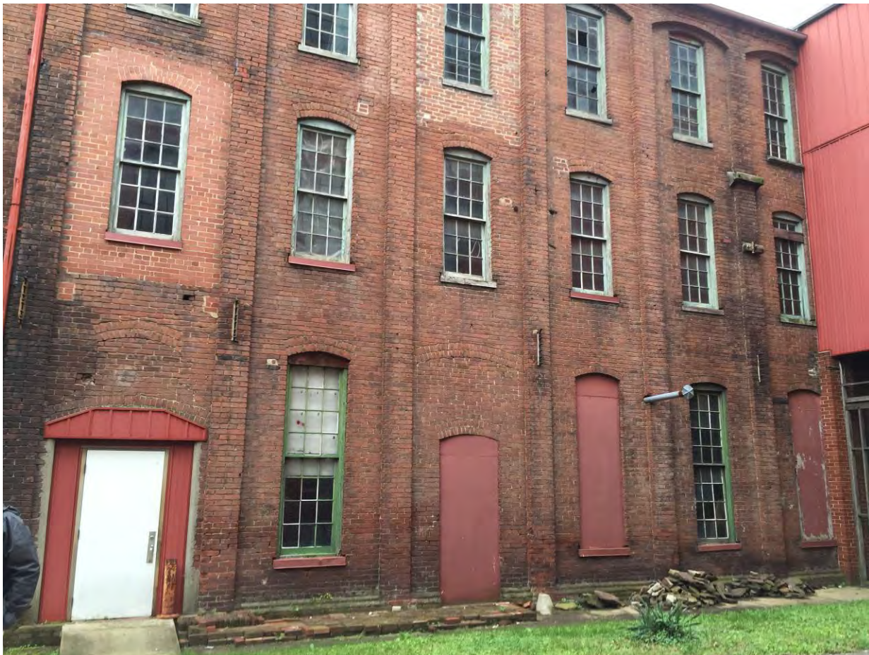
Photo 7. Enlarged view of east end of north elevation showing bricked in openings where the 1882 bridges were located, and 2 partially infilled openings in the 1 st and 3 rd bays from the left at ground level where finished goods were loaded on railcars from the packing room.
