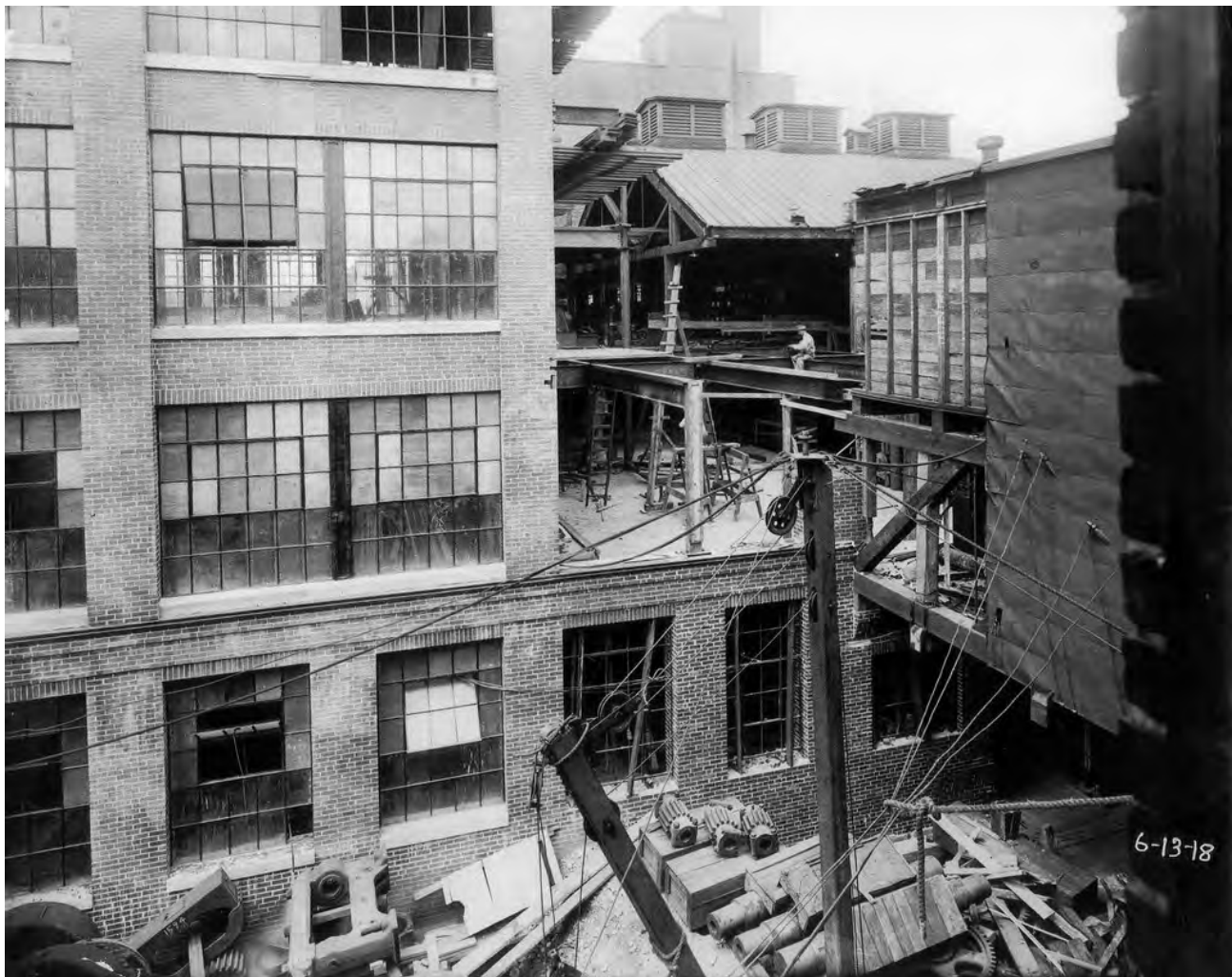
6-13-18 Construction photo of Building C under construction west of Building B, where the original vulcanizers were located. The south elevation of Building H is visible in the background above the ventilators on the roof of the vulcanizer building. The 2-story bridge in the left foreground will connect Building A to Building C after Building K, the new vulcanizer building on Rose Street is placed in service. Photo taken from Building A looking northeast. Image downloaded at http://www.lycoming.edu/textile/garment.html
