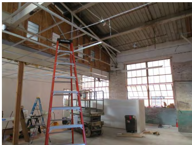
Photo 57. View of community kitchen under construction at northwest corner of the same space. Note operable sashes and open steel frame trusses.
