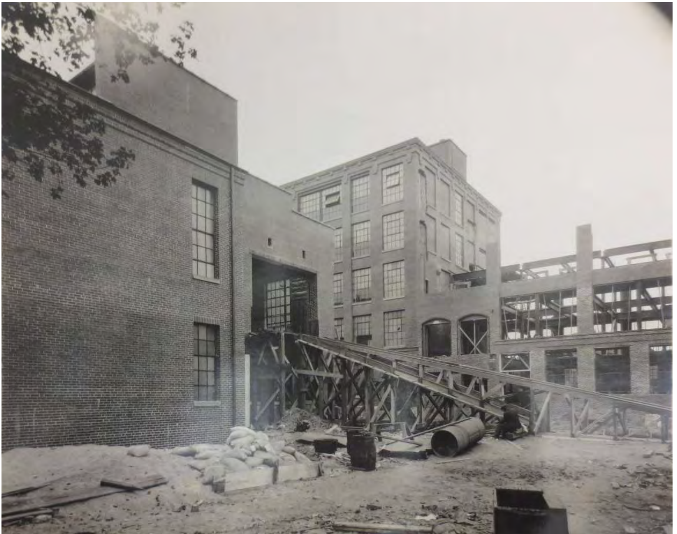
Circa 1918 Construction Photo of Building K (foreground), Building H (background center) and Building L (background right); Lycoming Rubber Company; looking southwest from Rose Street; Lockwood Greene Records, Archives Center, National Museum of American History, Smithsonian Institution
