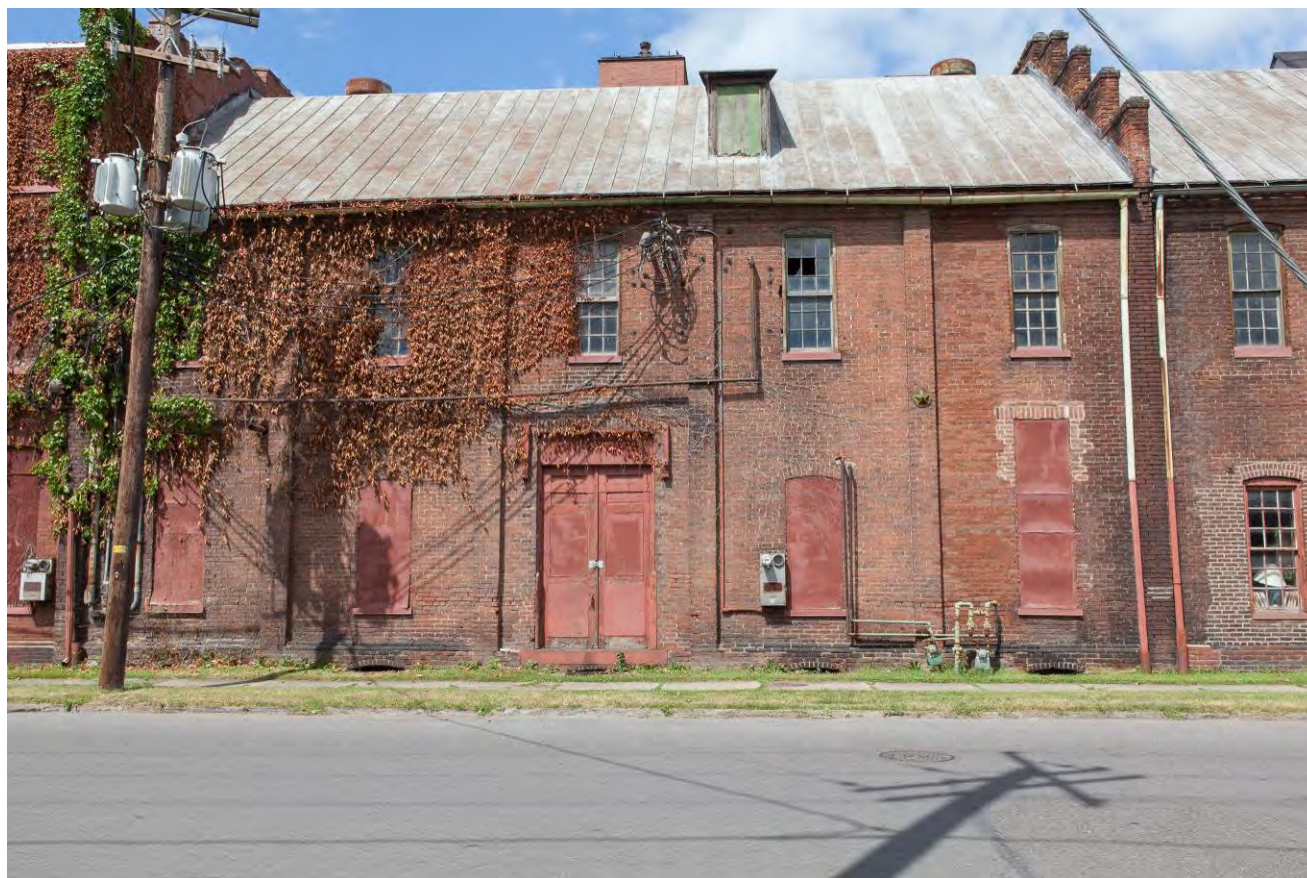
Photo 16. East elevation of the Rose Street façade of Building D between Building A and Building D extensions
