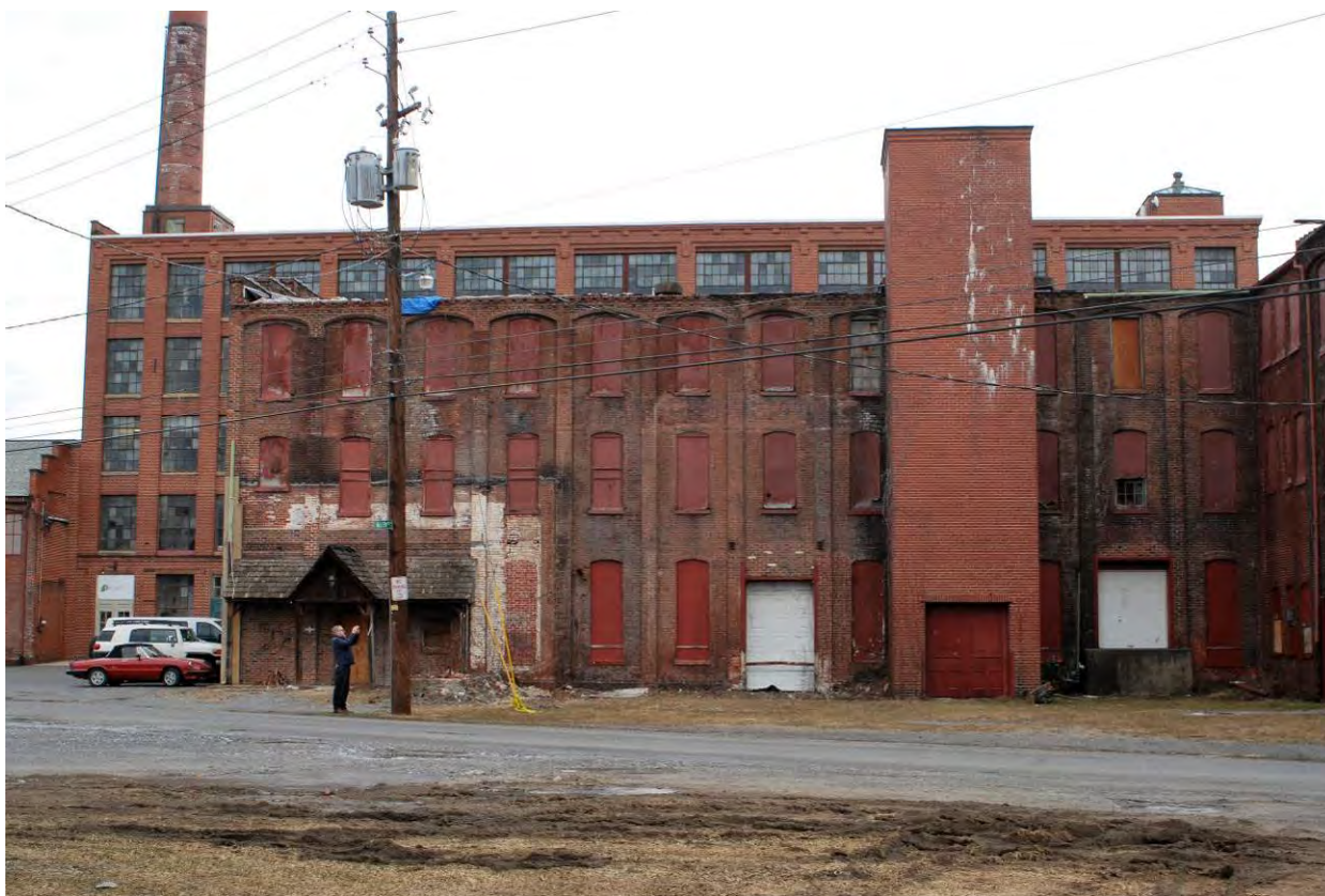
Photos 3. South Elevation of Building A west of Building F, with 1918 elevator tower.
