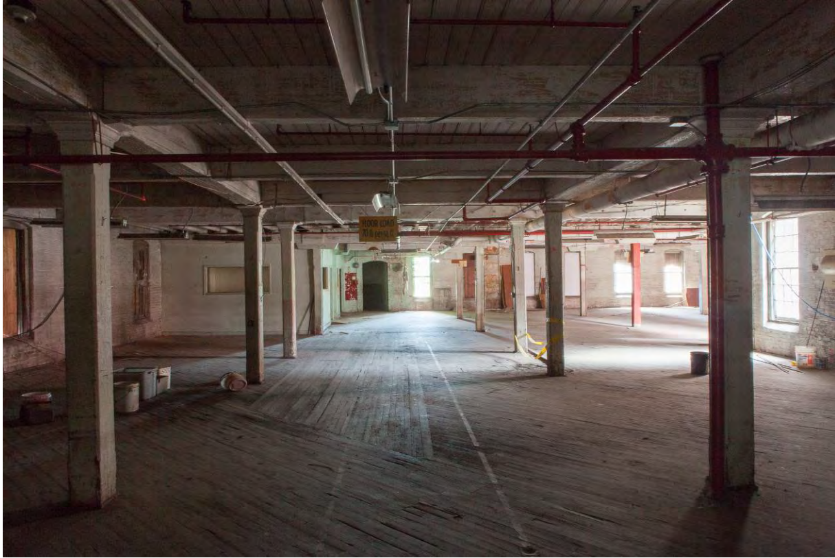
Photo 15. View of 2 nd floor of Building A extension looking south. Note the cast iron columns in the 4 bays of the foreground, and the timber frame structure in Building A in the 2 bays in the background.
