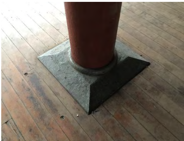
Photo 42. Original 22" by 22" by 3/4 "column base
