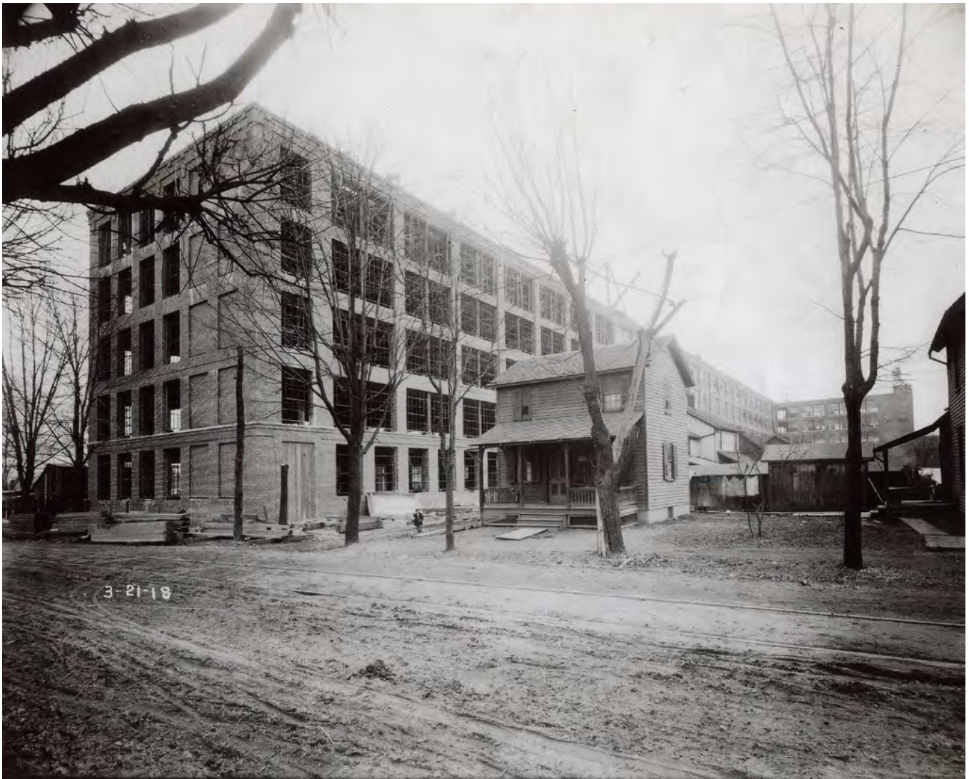
3-21-18 Construction photo of Building L immediately north of Building H, with Building C addition in background, taken from Park Avenue west of Allen Street. Image downloaded at http://www.lycoming.edu/textile/garment.html
