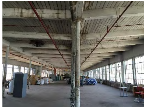
Photo 70. View of 5 th floor looking south. Note 5" cast iron rainwater conductor next to column.
