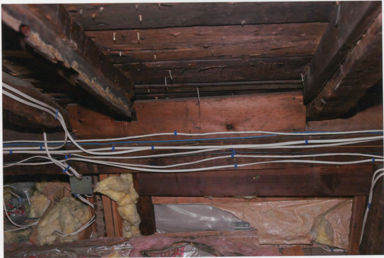
Photo 20. Enos Kellog House, Norwalk, Fairfield County, Connecticut. Attic, view east showing raised plate framing detail. July 29, 2011, Tod Bryant
