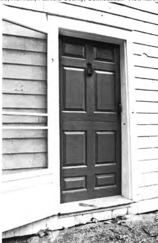
Photo 2. Enos Kellogg House, Norwalk, Fairfield County, Connecticut. View east showing original front door and hardware, July 29, 2011, Tod Bryant
