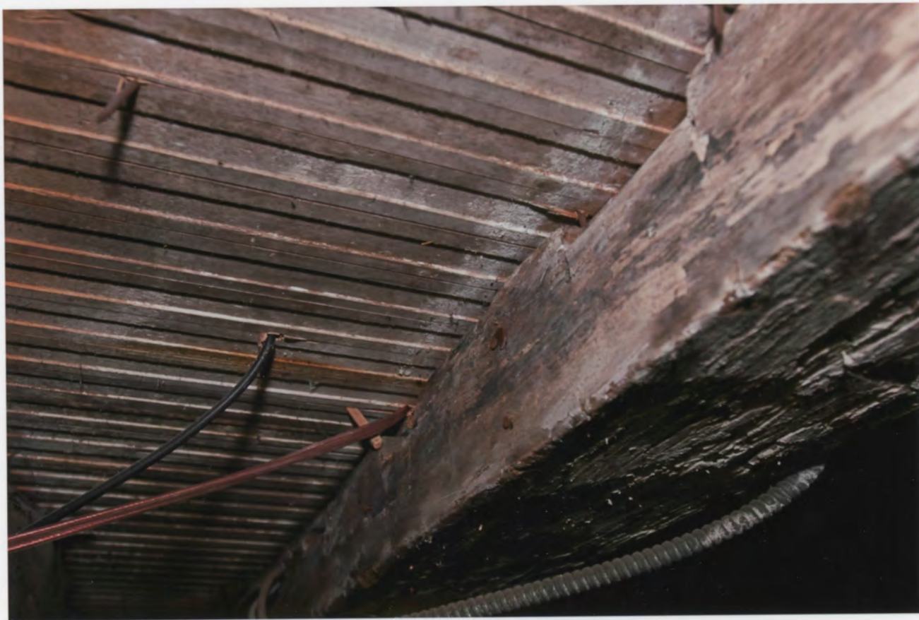
Photo 19. Enos Kellogg House, Norwalk, Fairfield County, Connecticut. Basement showing dust slits in floor joist. July 29, 2011, Tod Bryant
