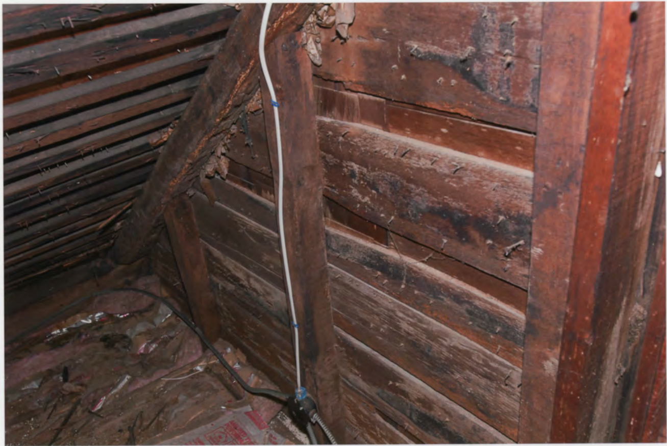
Photo 5. Enos Kellogg House, Norwalk, Fairfield County, Connecticut. Attic showing original siding used as sheathing. July 29, 2011, Tod Bryant
