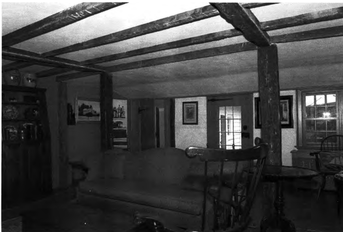
Photo 13. Enos Kellogg House, Norwalk, Fairfield County, Connecticut. First floor interior view northeast showing framing July 29, 2011, Tod Bryant
