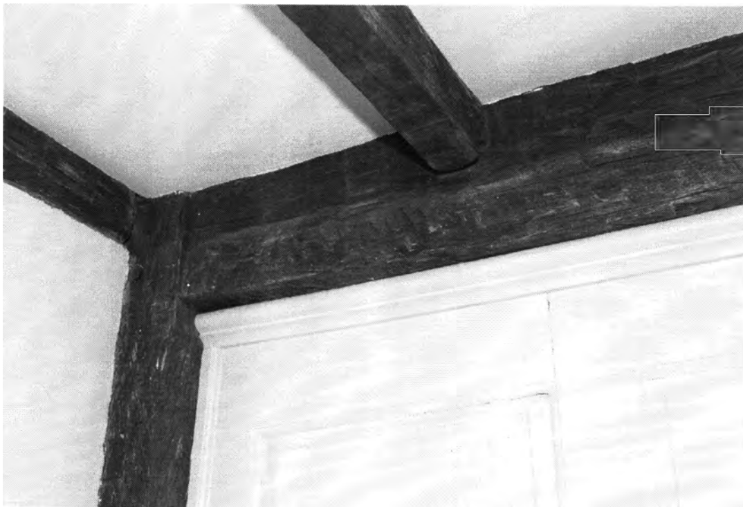
Photo 10. Enos Kellogg House, Norwalk, Fairfield County, Connecticut. First floor North Room, view southeast showing paneling and framing detail. July 29, 2011, Tod Bryant
