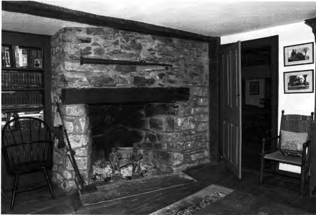
Photo 7. Enos Kellogg House, Norwalk, Fairfield County, Connecticut. First floor interior view northeast showing hall fireplace, framing and original interior door. July 29, 2011, Tod Bryant
