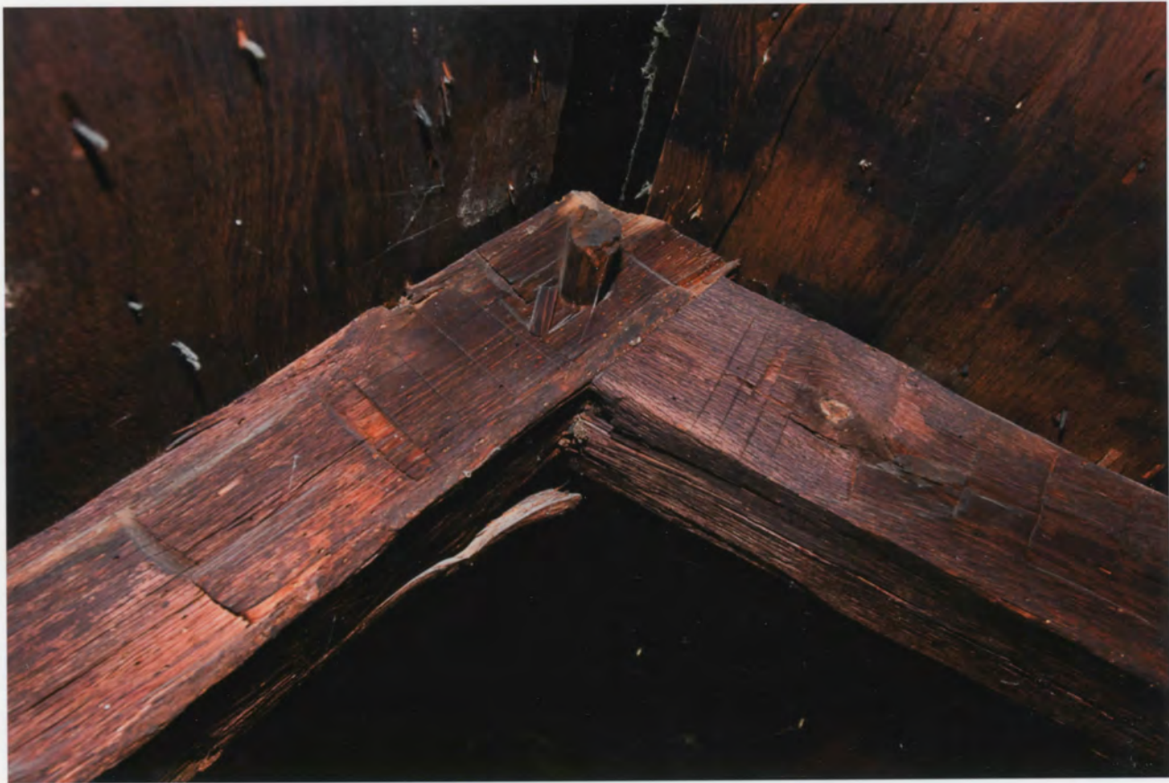
Photo 6. Enos Kellogg House, Norwalk, Fairfield County, Connecticut. Attic showing rafter framing detail and raising marks. July 29, 2011, Tod Bryant
