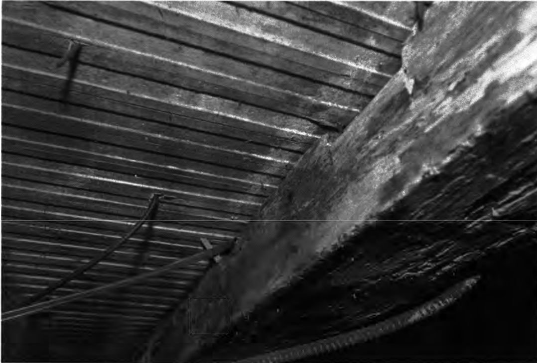
Photo 19. Enos Kellogg House, Norwalk, Fairfield County, Connecticut. Basement showing dust slits in floor joist. July 29, 2011, Tod Bryant
