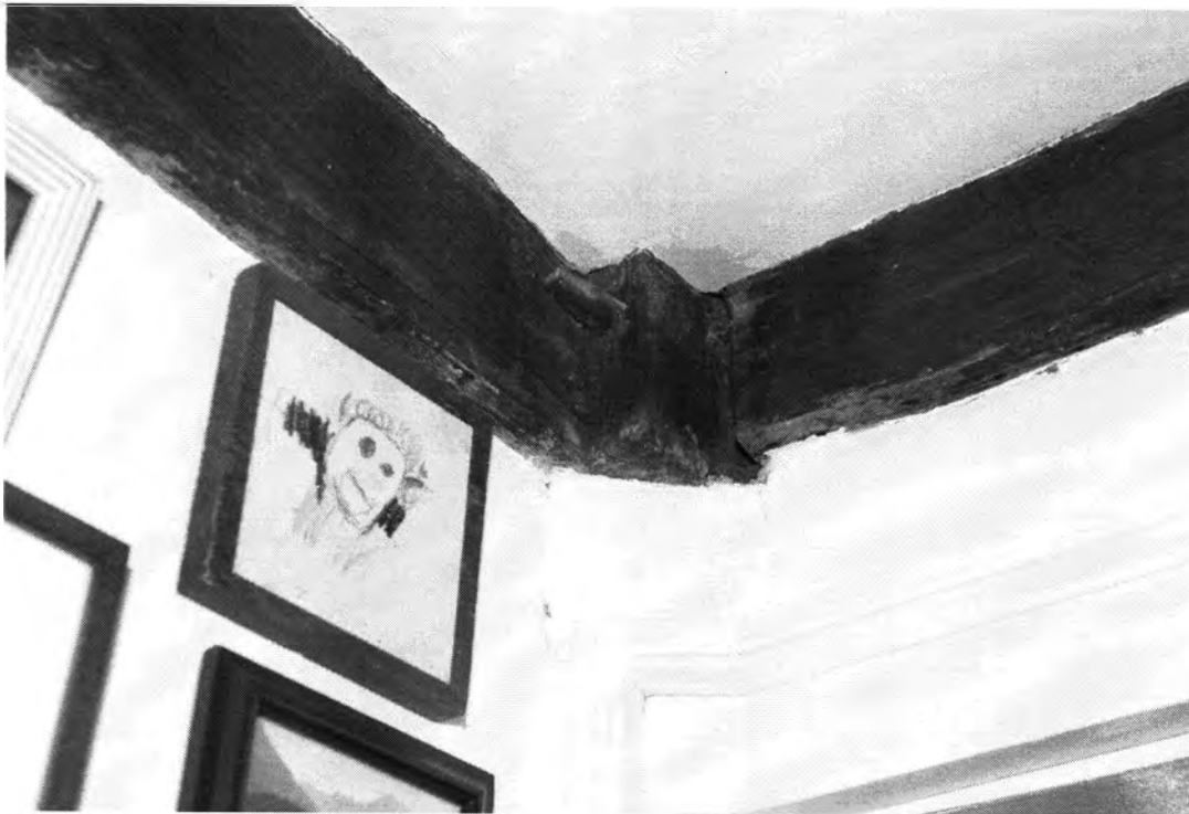
Photo 9. Enos Kellogg House, Norwalk, Fairfield County, Connecticut. First floor North Room, view northeast showing framing detail. July 29, 2011, Tod Bryant
