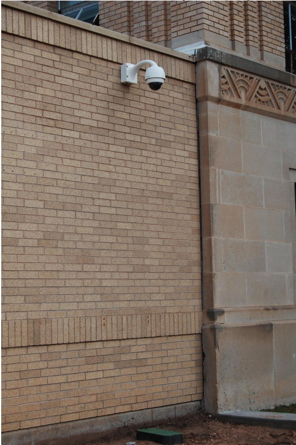
Photo 12: North Elevation where the Lubbock County Detention Facility meets the Lubbock County Jail
