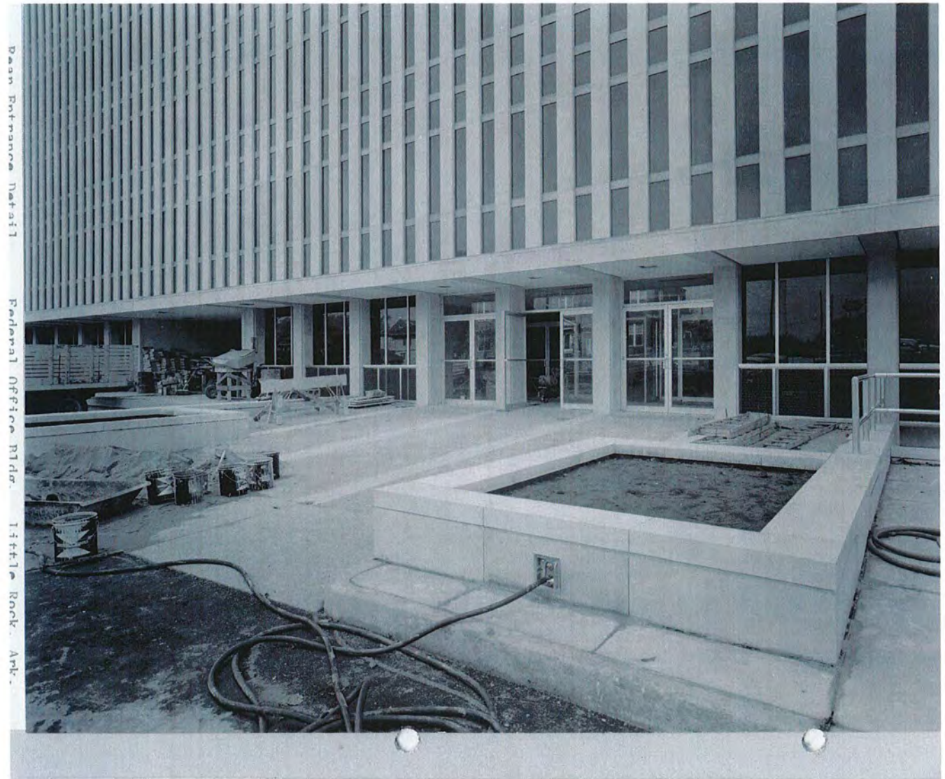
Rear entrance detail, Federal Building, Little Rock, AR (GSA EDOCs Photo 14030; Photo dated November 1, 1961).
