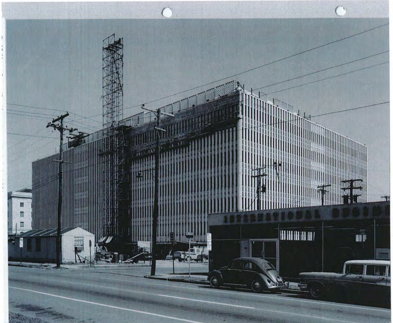
Federal Building (under construction), Little Rock, AR (GSA EDOCs Photo 14025; Photo dated June 1, 1961).
