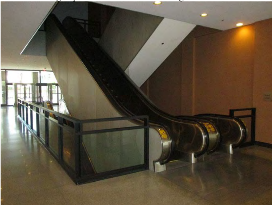
TX_Dallas County_One Main Place_0014 West escalator group at first floor – camera facing northeast
