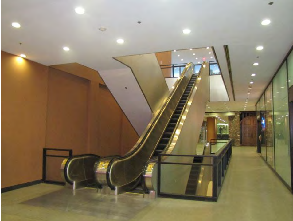
TX_Dallas County_One Main Place_0017 East escalator group at plaza level – camera facing northwest
