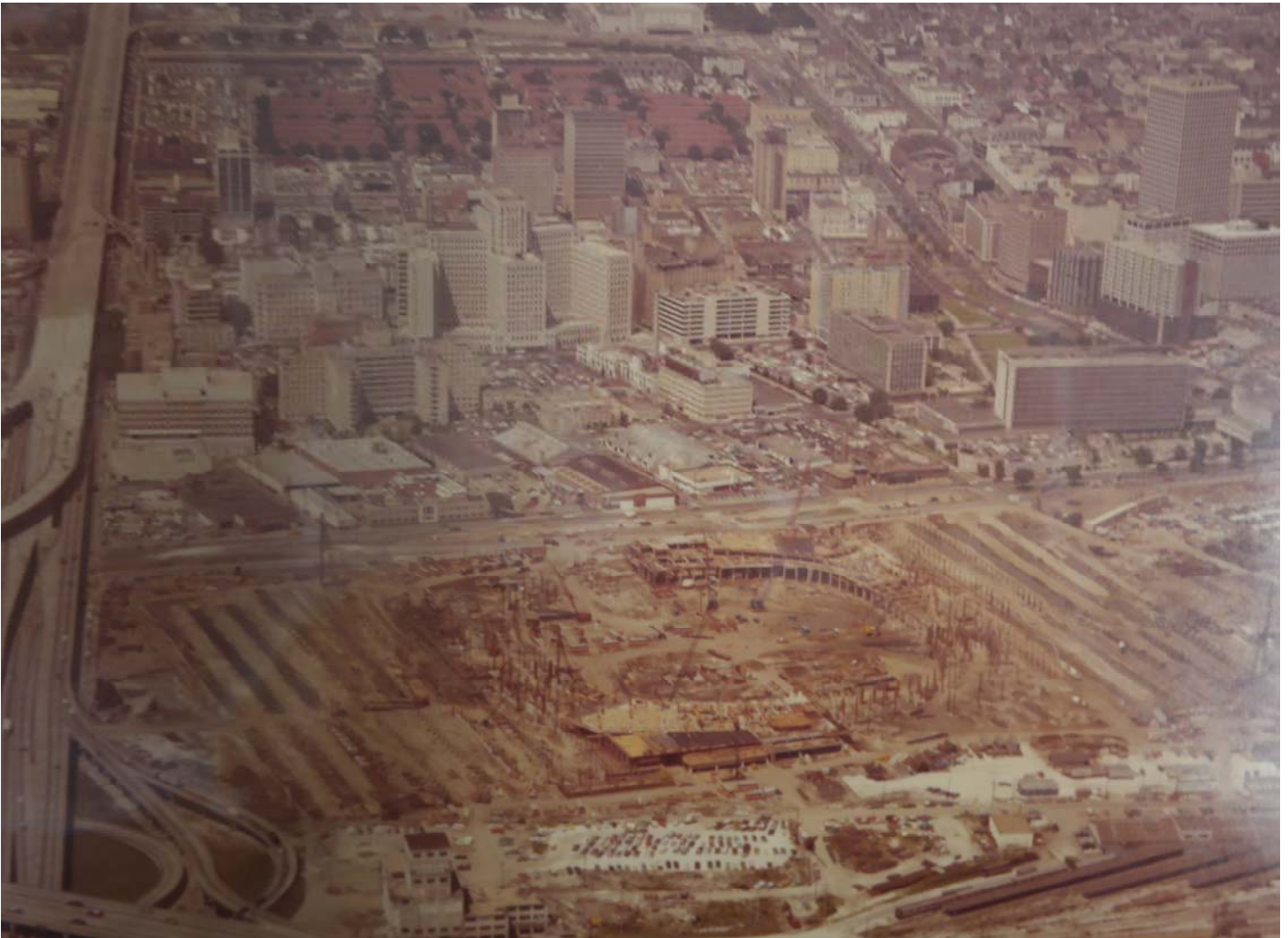
Figure 18. Aerial view of construction; Source: Curtis and Davis Office Records, Southeastern Architectural Archives, Tulane University
