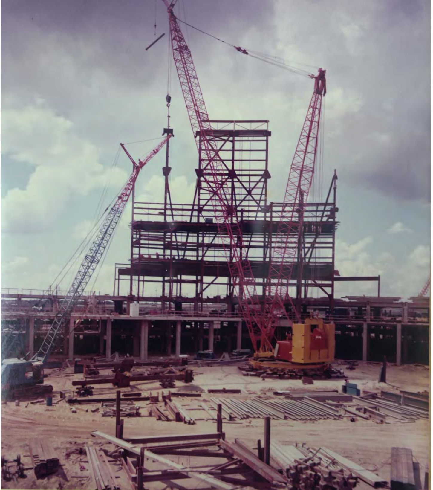
Figure 17. Construction photo of pilings and walls; Source: Curtis and Davis Office Records, Southeastern Architectural Archives, Tulane University
