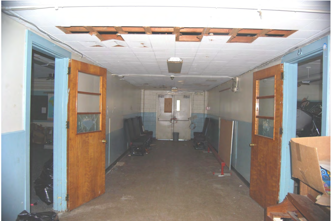
H-13. Looking W in ground floor corridor, 1952 addition; the exterior doors in center of photo now connect to the 2013 addition
