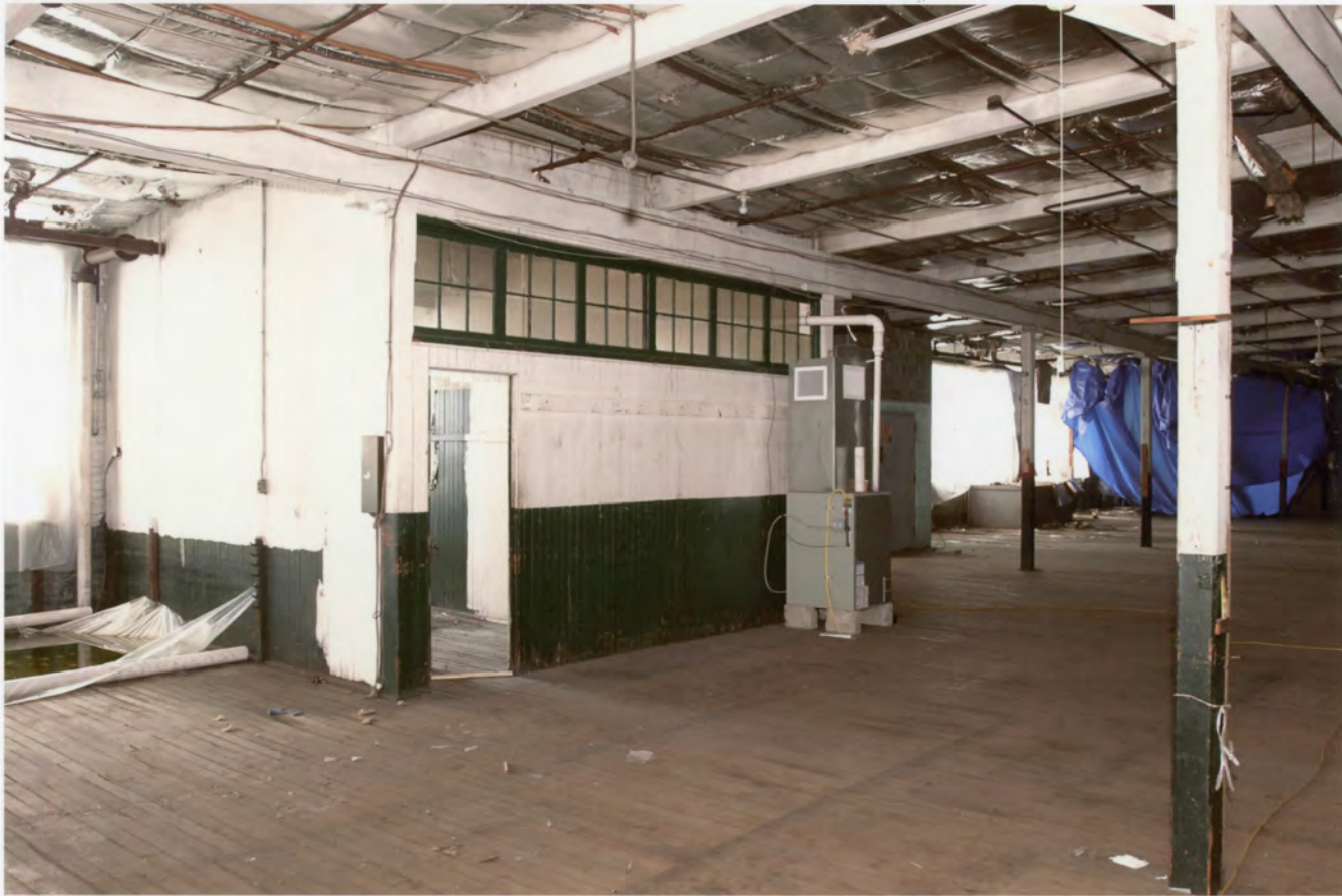
Photo 15. Le Roy Shirt Co., Norwalk, Fairfield County, Connecticut. Second floor interior view southwest showing locker room. August 5, 2011 Tod Bryant
