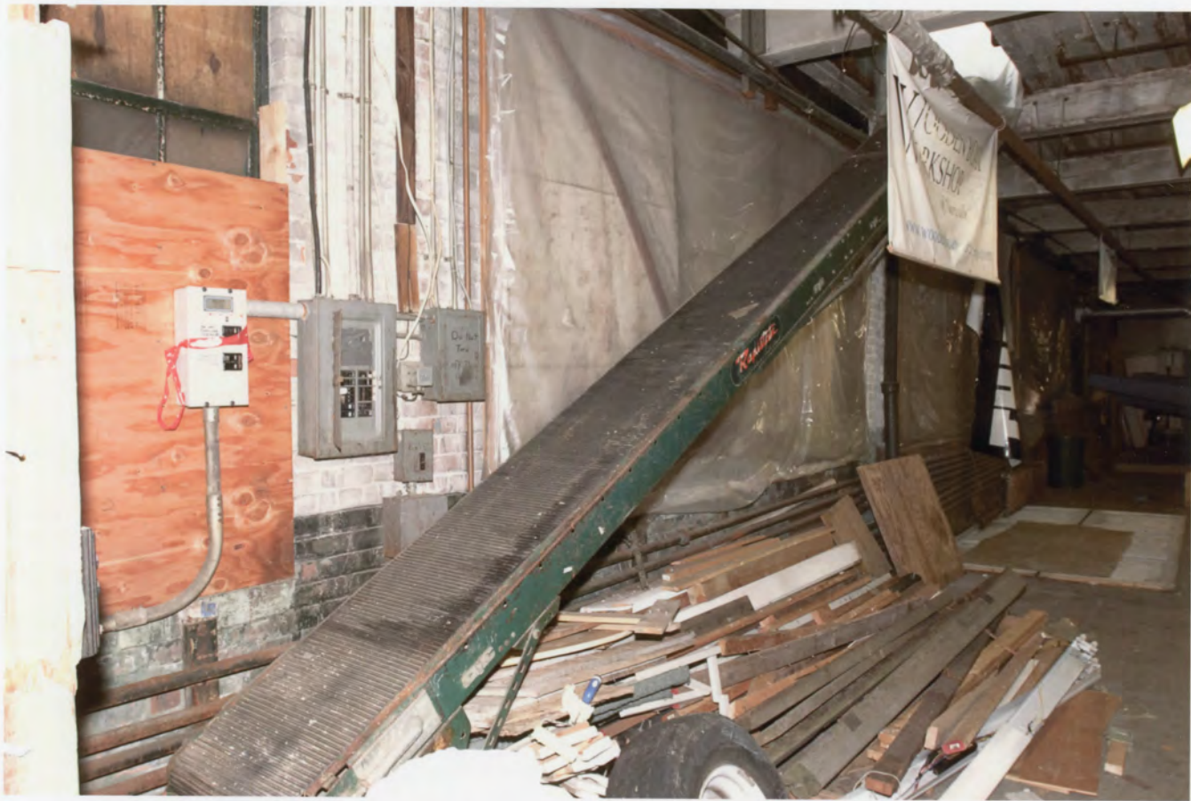
Photo 12. Le Roy Shirt Co., Norwalk, Fairfield County, Connecticut. First floor interior view southwest showing front conveyor. August 5, 2011 Tod Bryant
