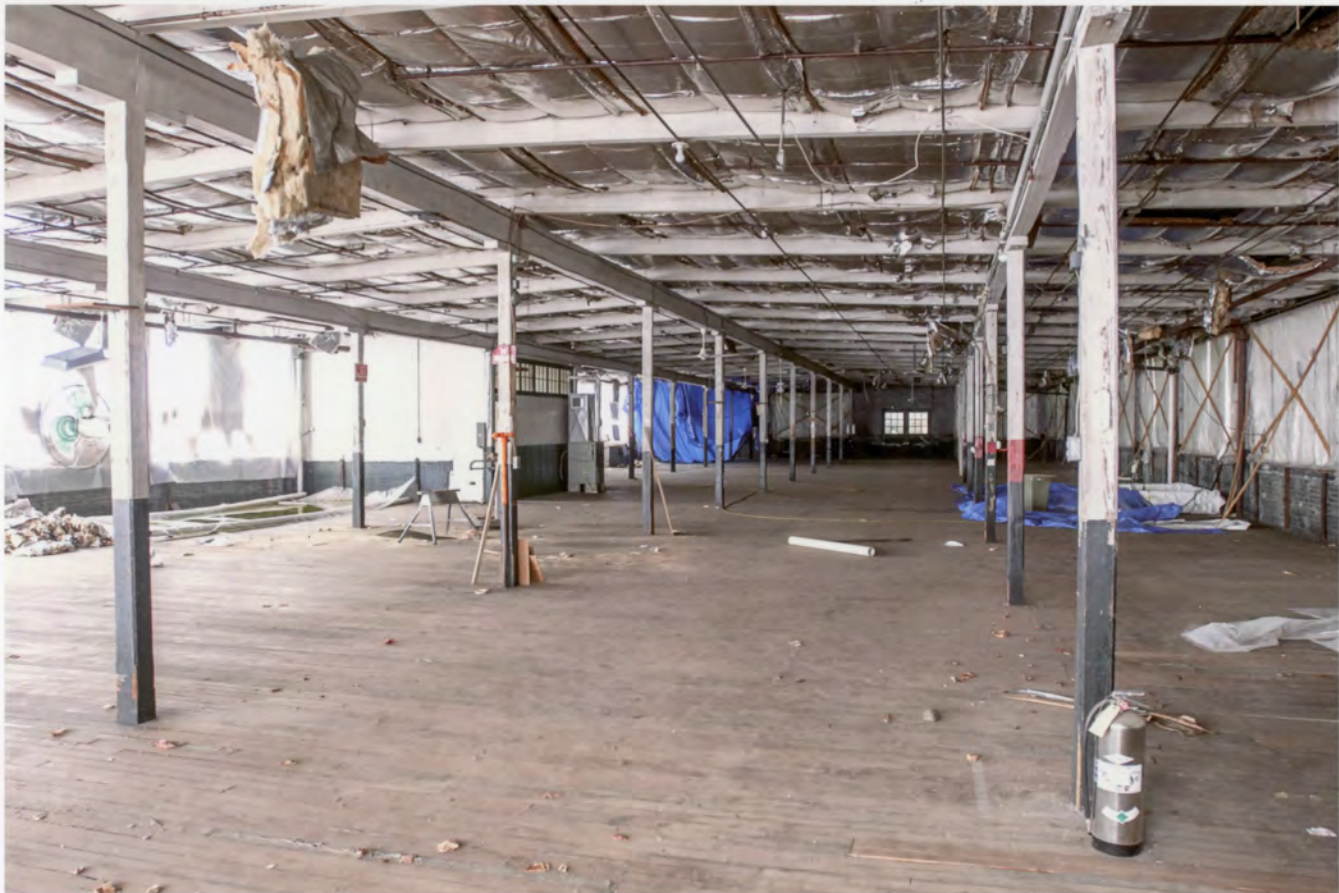
Photo 13. Le Roy Shirt Co., Norwalk, Fairfield County, Connecticut. Second floor interior view west. August 5, 2011 Tod Bryant.
