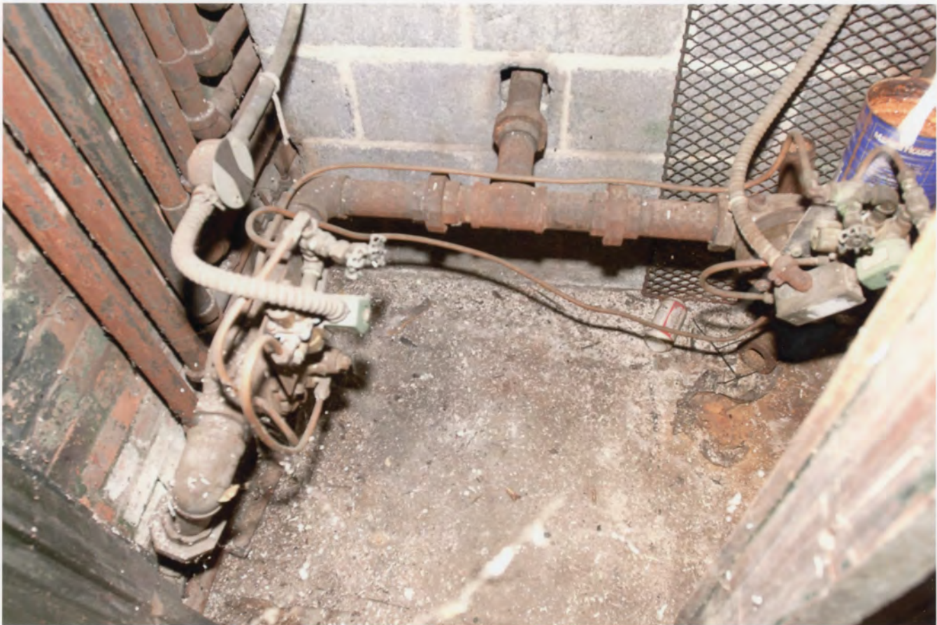
Photo 8. Le Roy Shirt Co., Norwalk, Fairfield County, Connecticut. First floor interior showing valves for water-powered elevator. August 5, 2011 Tod Bryant
