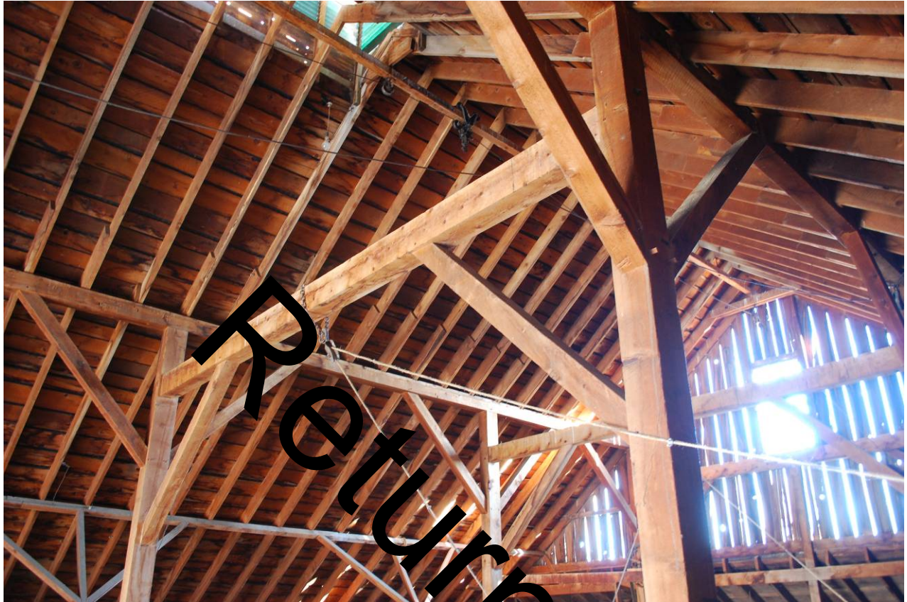
Photograph 6 – Barn interior, viewing primary framing and roof structure, looking up and southeast.
