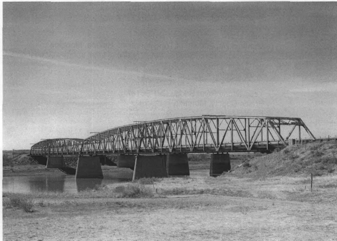
Photograph 0001. Yellowstone River Bridge. South profile and east portal. View to the northwest.
