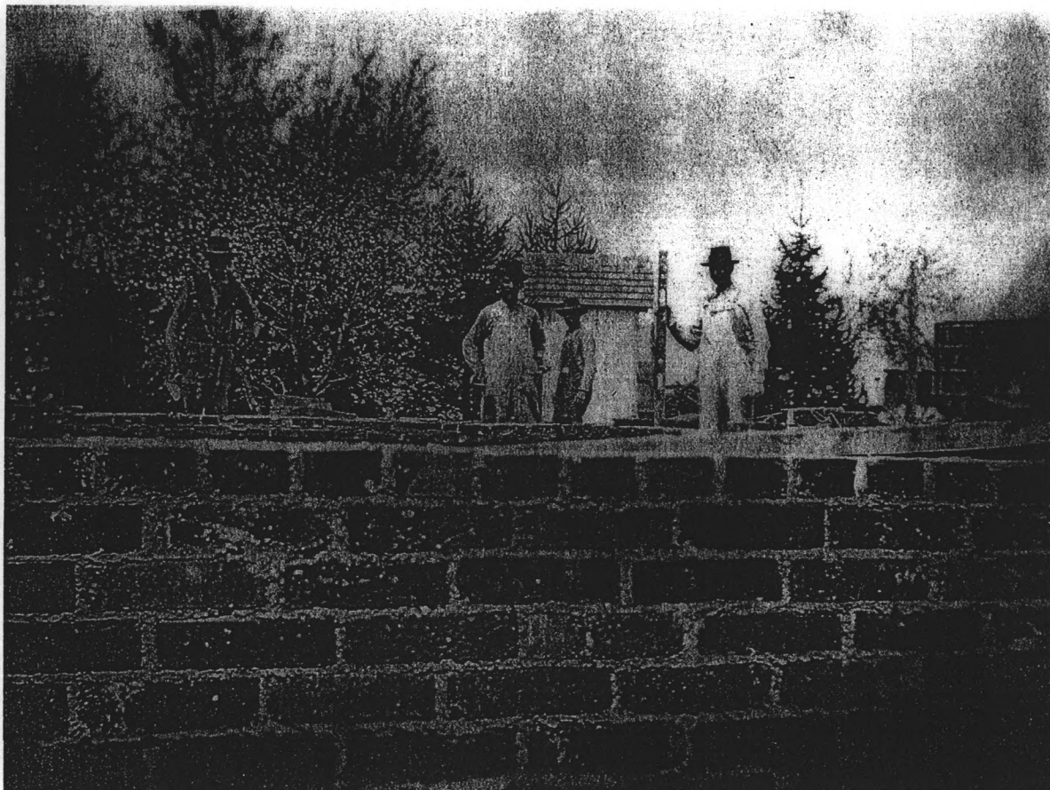
Douwe Sjaardema (front and center) and his crew pause while constructing the basement of the Vander Wilt Farmhouse. Douwe's crew included his sons and his brother Fred, who owned the Leighton Lumber Yard. The wood stave water tank shows at the right and a privy at center.
