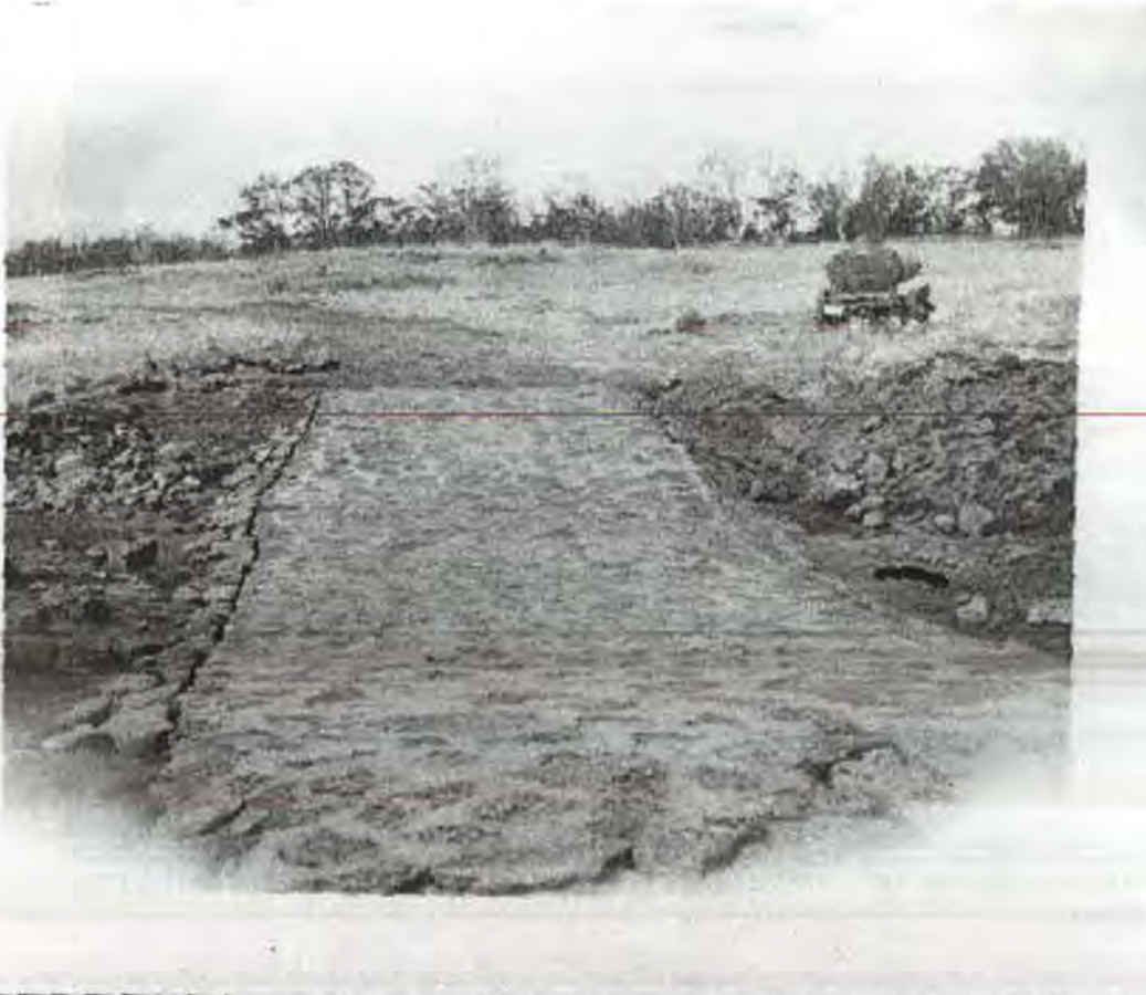
Fig. 2. Hilina Pali Ford #3 damaged from water flow due to heavy rains. Photographed by Frank Oberhansley, Feb. 1950. Source: Historic Photo Collection, HAVO 554, Binder 2 of 5, HAVO Archives.
