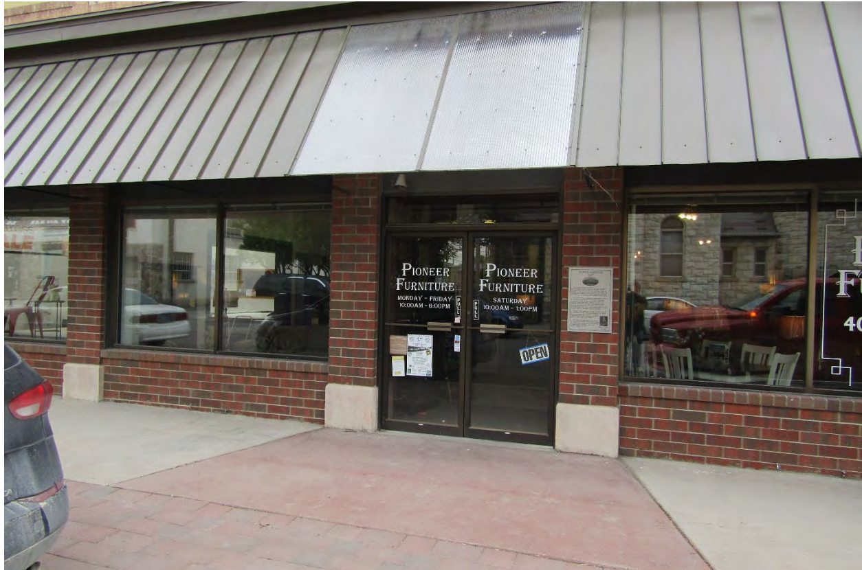
Description and view of camera: Andrus Hotel. Remodeled primary entry on southwest (west) façade. View to northeast. MT_BeaverheadCounty_AndrusHotel_0011
