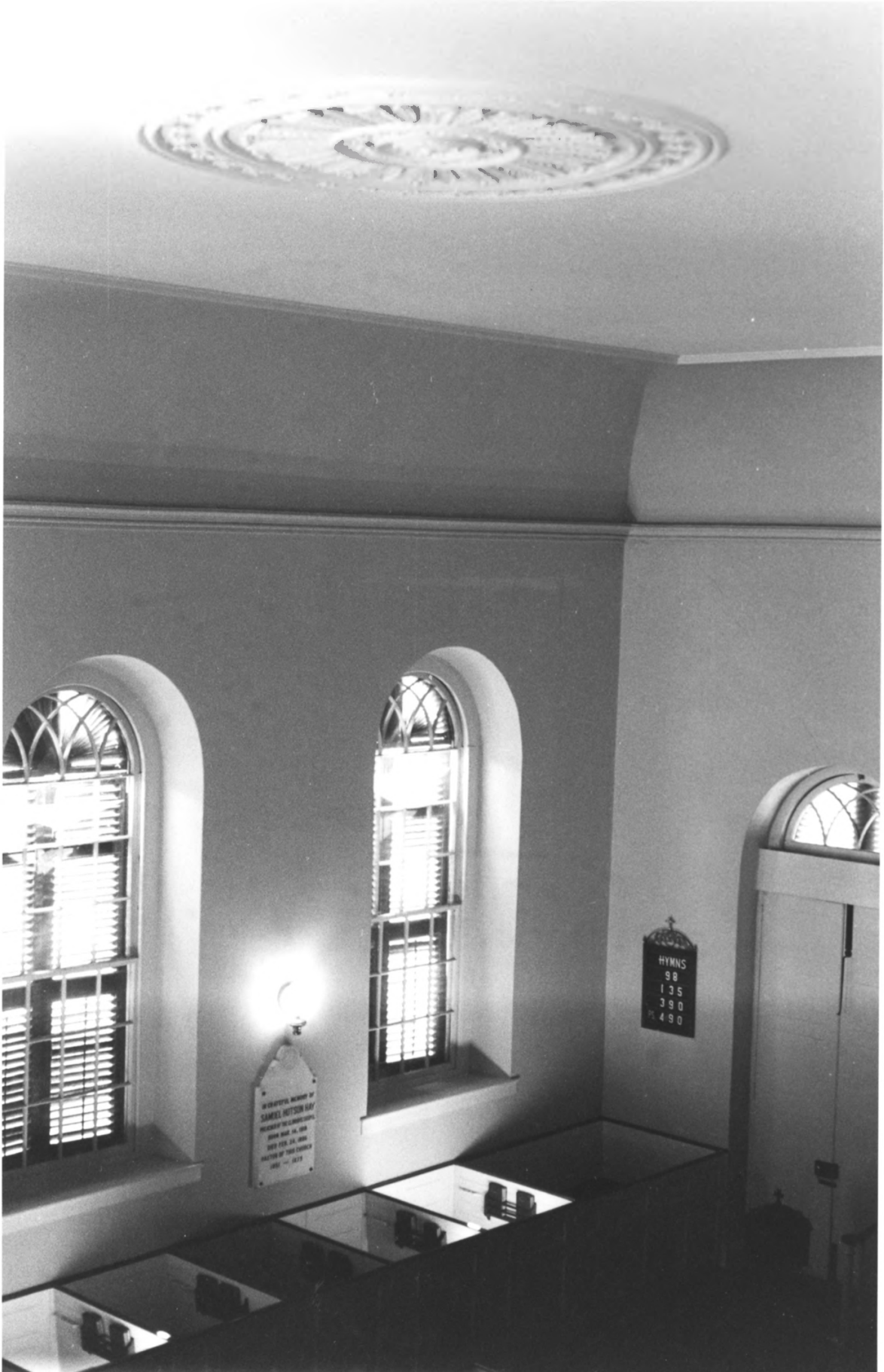
Bethesda Presbyterian Church Kershaw County, South Carolina 5/31/84 Interior: view of medallion, East & South Facades
