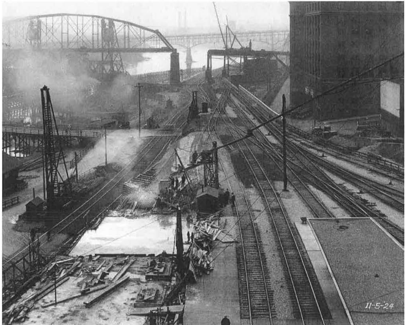
1924: Deck construction, west of Waiting Room, looking west (Image courtesy of the Elon Piche Collection, Ramsey County Regional Railroad Authority)
