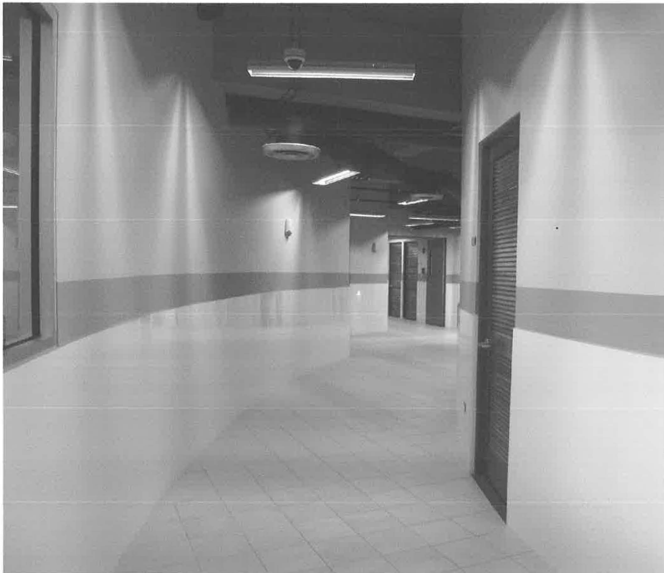
Fig. 5. Part of the area from the old warehouse rehabilitated to make space for classrooms, service rooms and lunch area in the first floor. The entire intervention was done in the space behind the walls where the murals are located.
