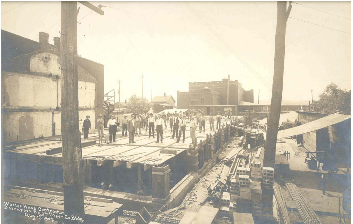
Early construction, August 19, 1907, looking south. Train cars visible directly south of building. (Source: Valley Construction Company, April 2014)
