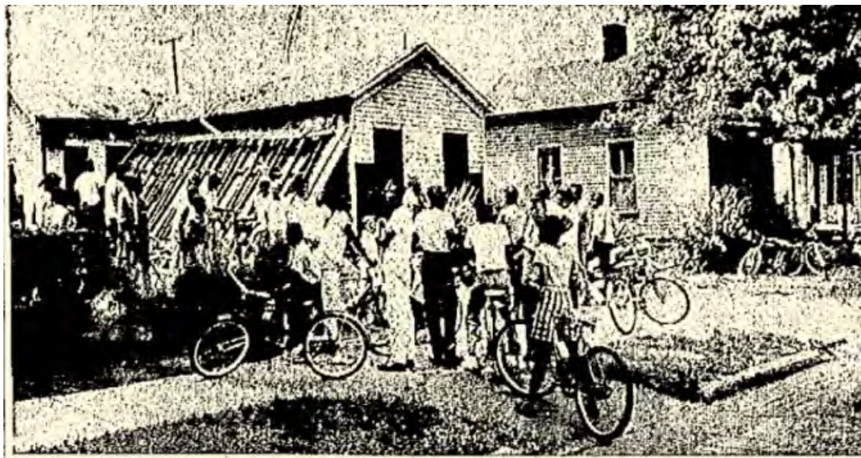
Figure 7: North End children await the demolition of two homes for the McKinley Pool ( Portsmouth Times ).
