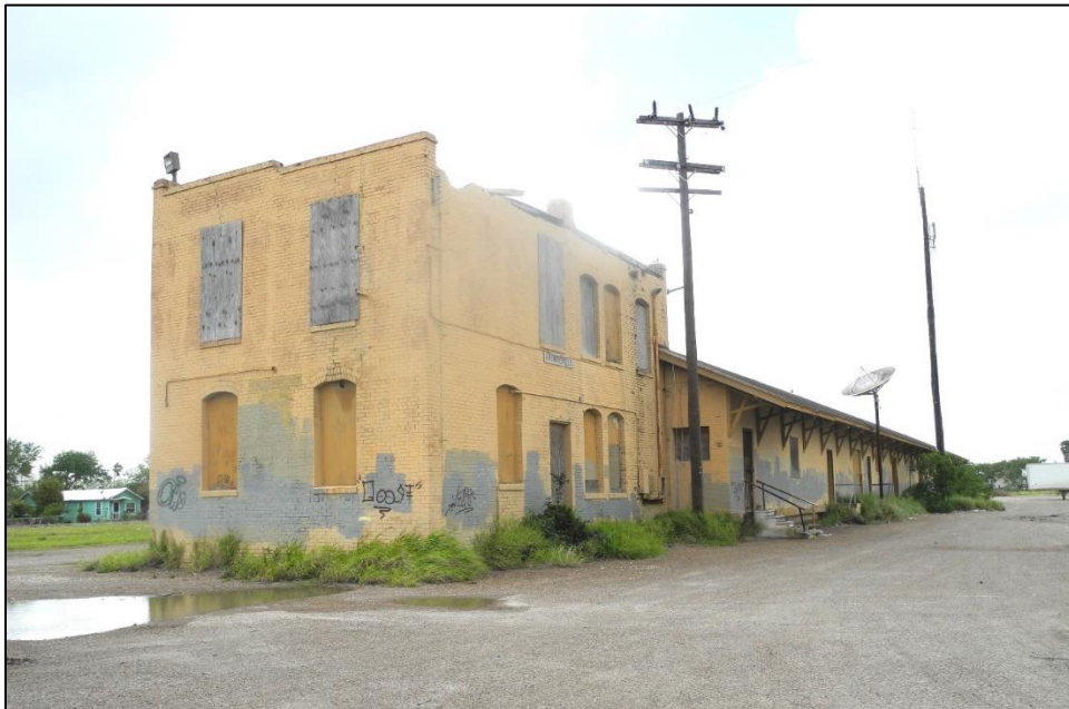
PHOTO 2: St. Louis, Brownsville & Mexico Railway Co. Depot Office (left) and Freight Depot (right), (Resources 2 and 1), side/east and rear/north elevations, facing northwest.
