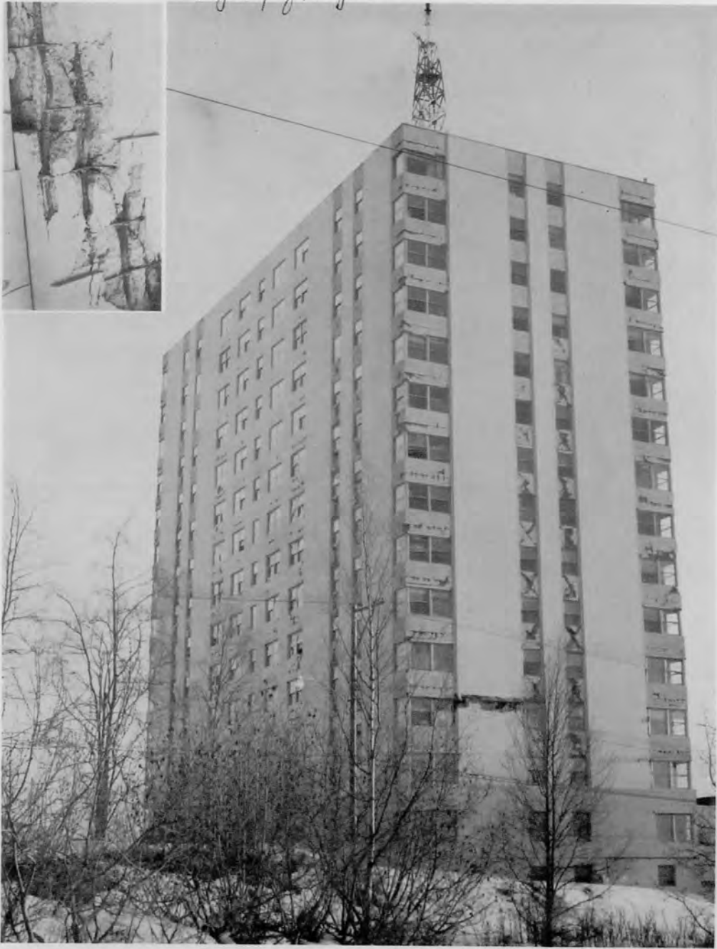
The Mt. McKinley Apartment Building stands empty and forelorn. Insert (Huntsman Photo) shows a portion of the outer facing torn away and the twisted reinforcing steel.
