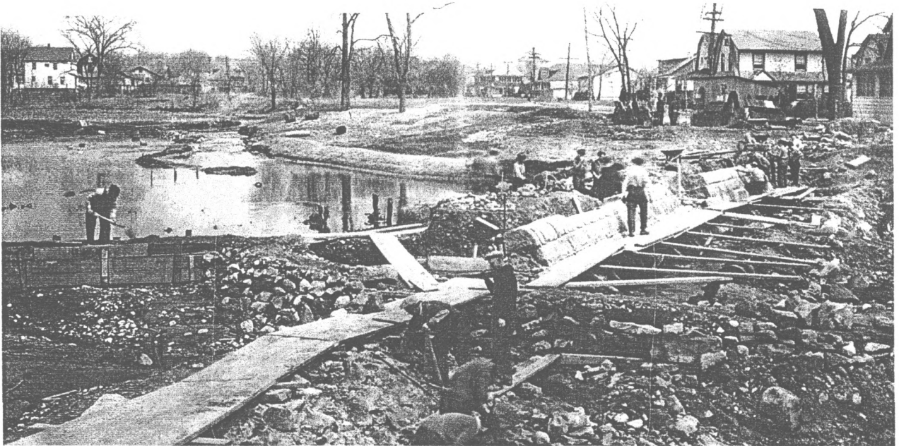
Photo H-23: Arnold Dam on Van Winkle Pond under construction ca. 1936. Source: H. S. Dutcher, Photograph Album compiled for the Passaic County Park Commission (1935-1940). Files of the Passaic County Parks Department, Paterson, NJ.
