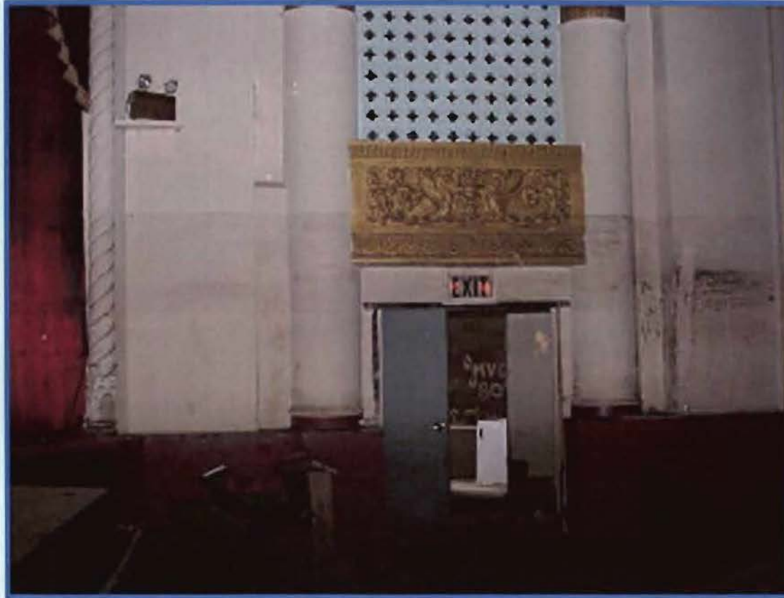
1999 Hurricane Floyd flood water level at lowest point of auditorium
