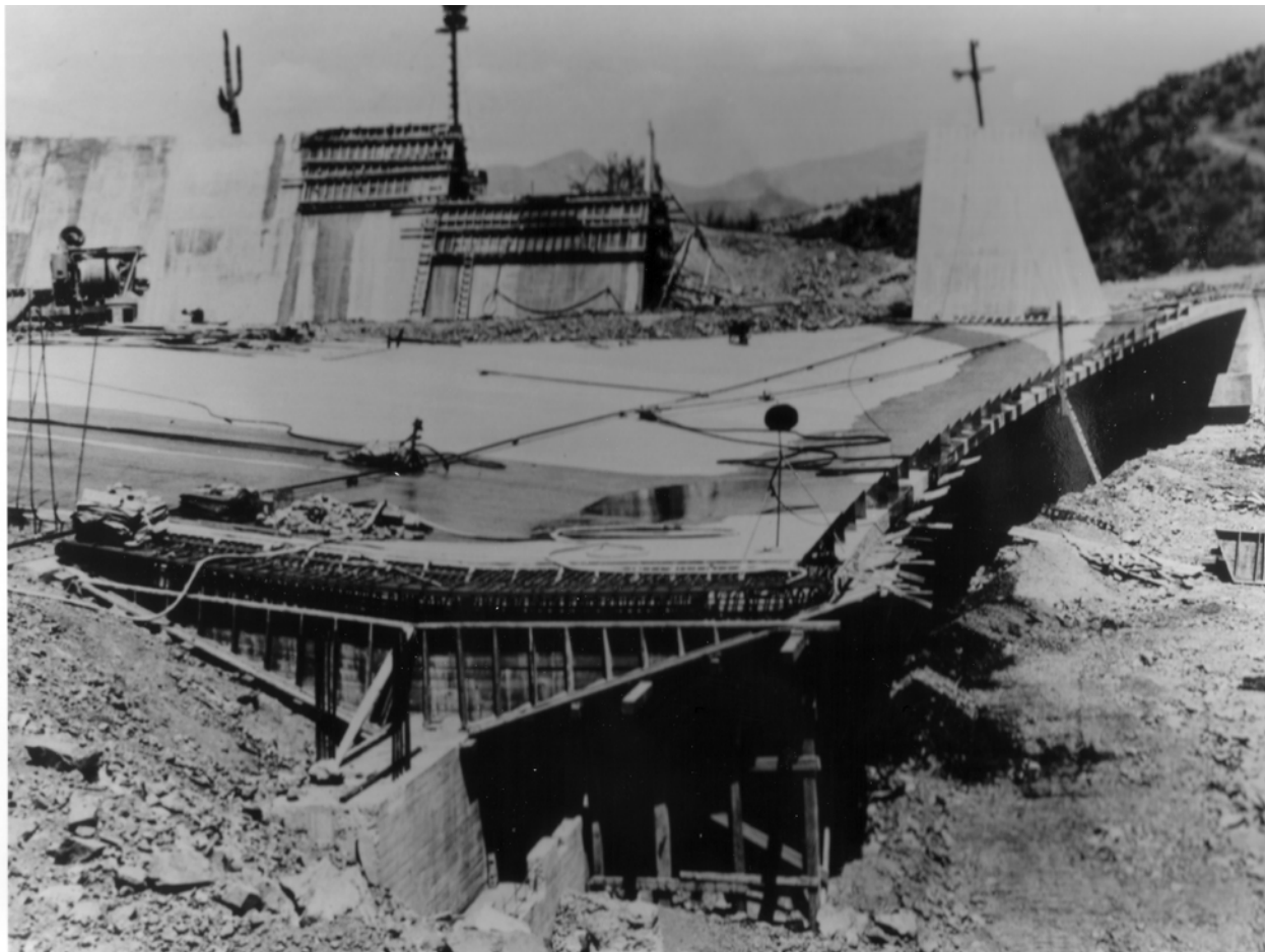
Historic Photo 8. Construction of the left spillway sidewall at Horseshoe Dam. Photo taken on June 8, 1945.
