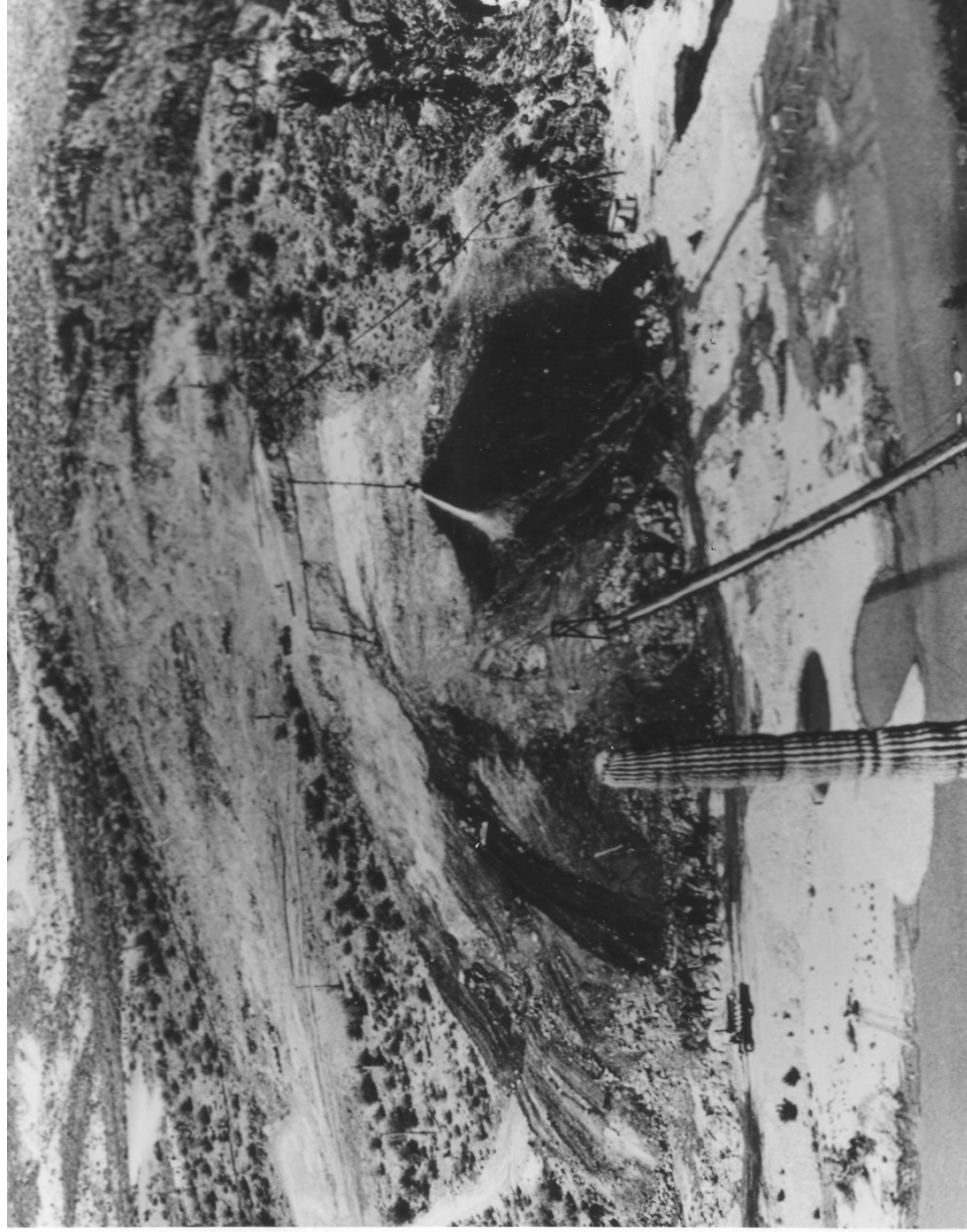
PHOTO No. AZ-24-32 VIEW FROM POINT "A" DURING CLEANING AND SLUICING OF WEST ABUTMENT. SITE OF SPILLWAY CHANNEL ALSO CLEARED. 29 August 1944.
