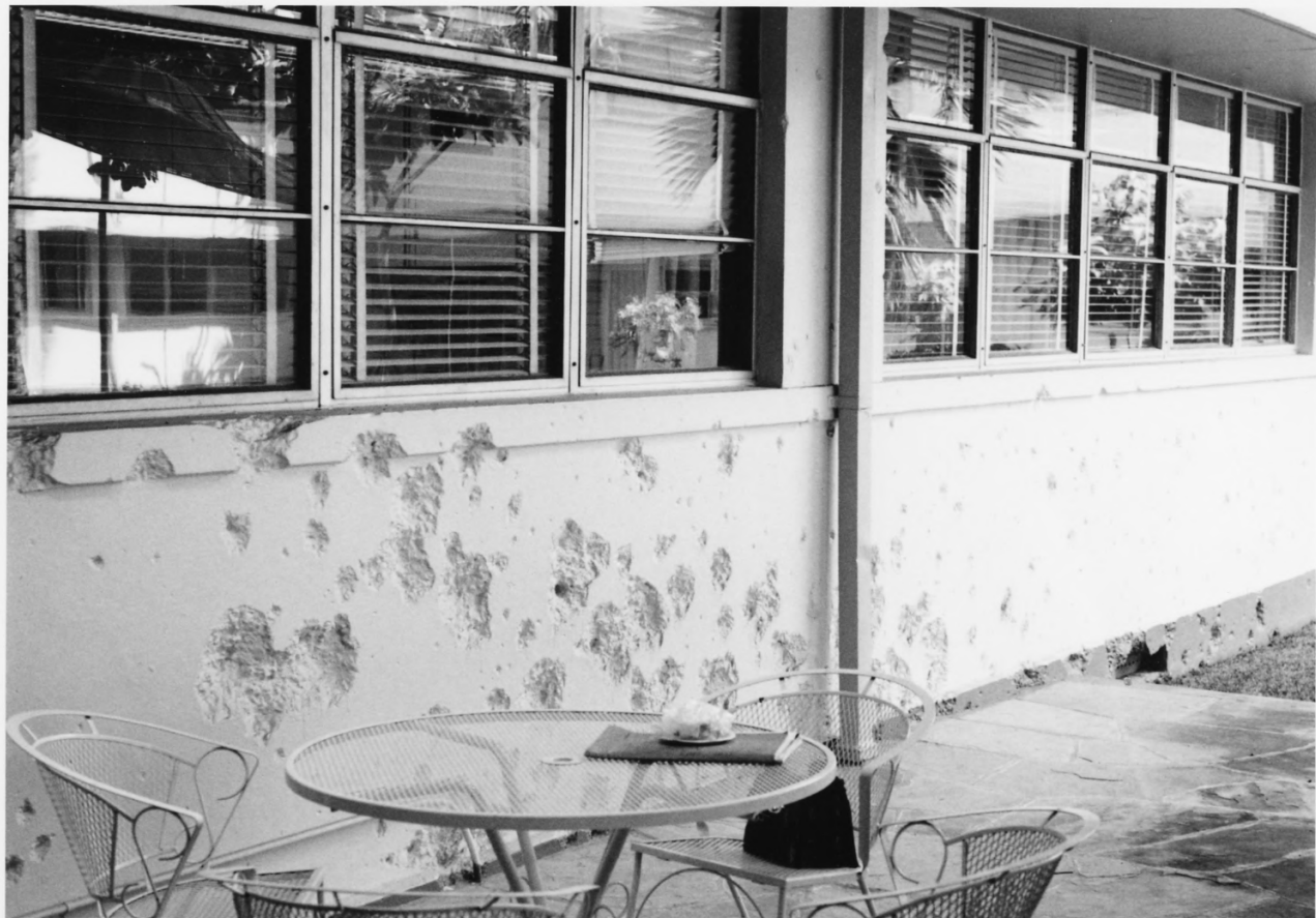
6. Bullet holes still pockmark the barracks' walls. The structure now is an administrative building.
