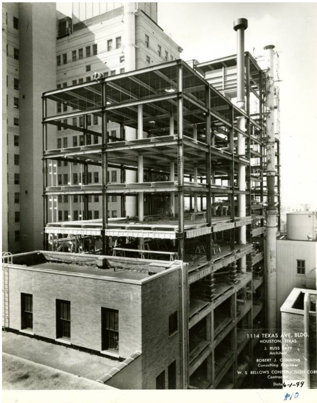
South view of 1114 Texas Avenue under construction, c.1949. The building in the foreground is the SWB Capitol Central Office Building.
