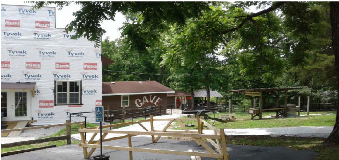
Figure 22: c.1960 Caretaker's Cabin with 2017 construction, Non-Contributing Building. Image taken by Kevin Bright, Summer 2017.
