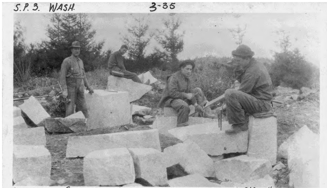
SPLITTING GLACIAL GRANITE FOR CARETAKER'S HOUSE. Splitting granite for Caretaker's Residence (ID#1) chimney.
