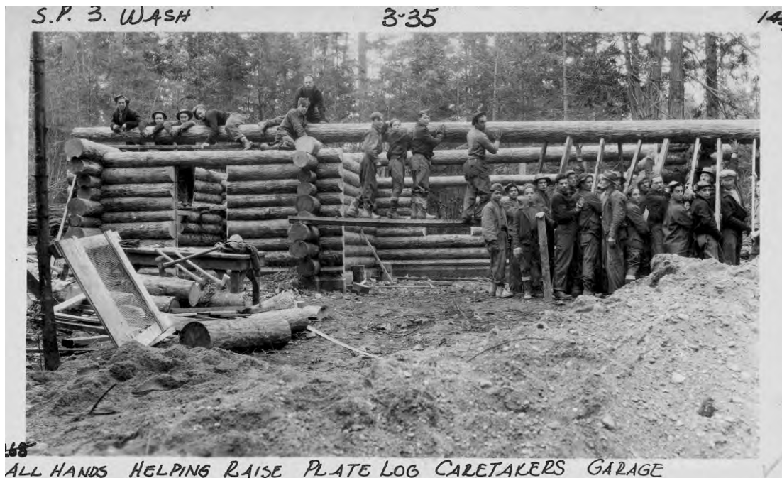
266 CARETAKER'S GARAGE SHOWING LOGWALL CONSTRUCTION Constructing log walls at Caretaker's Shop and Garage (ID#2), view to south.
