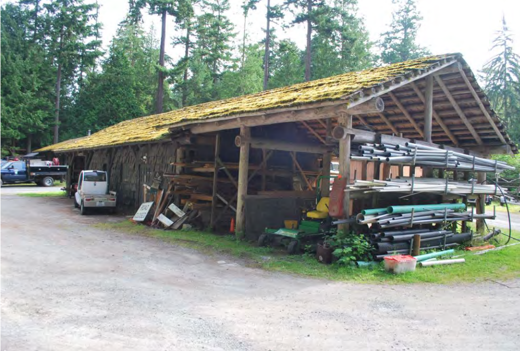
Photo 6 of 8: Cranberry Lake Maintenance Shop (ID#3), view to northeast showing south addition, taken 8/1/2012.
