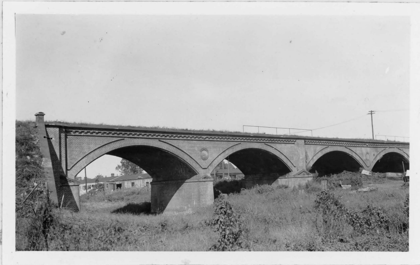
Bridge Central of Georgia, Ry. 1858. Crossing Ogeechee Canal west of yards near Louisville Road and Canal Street.
