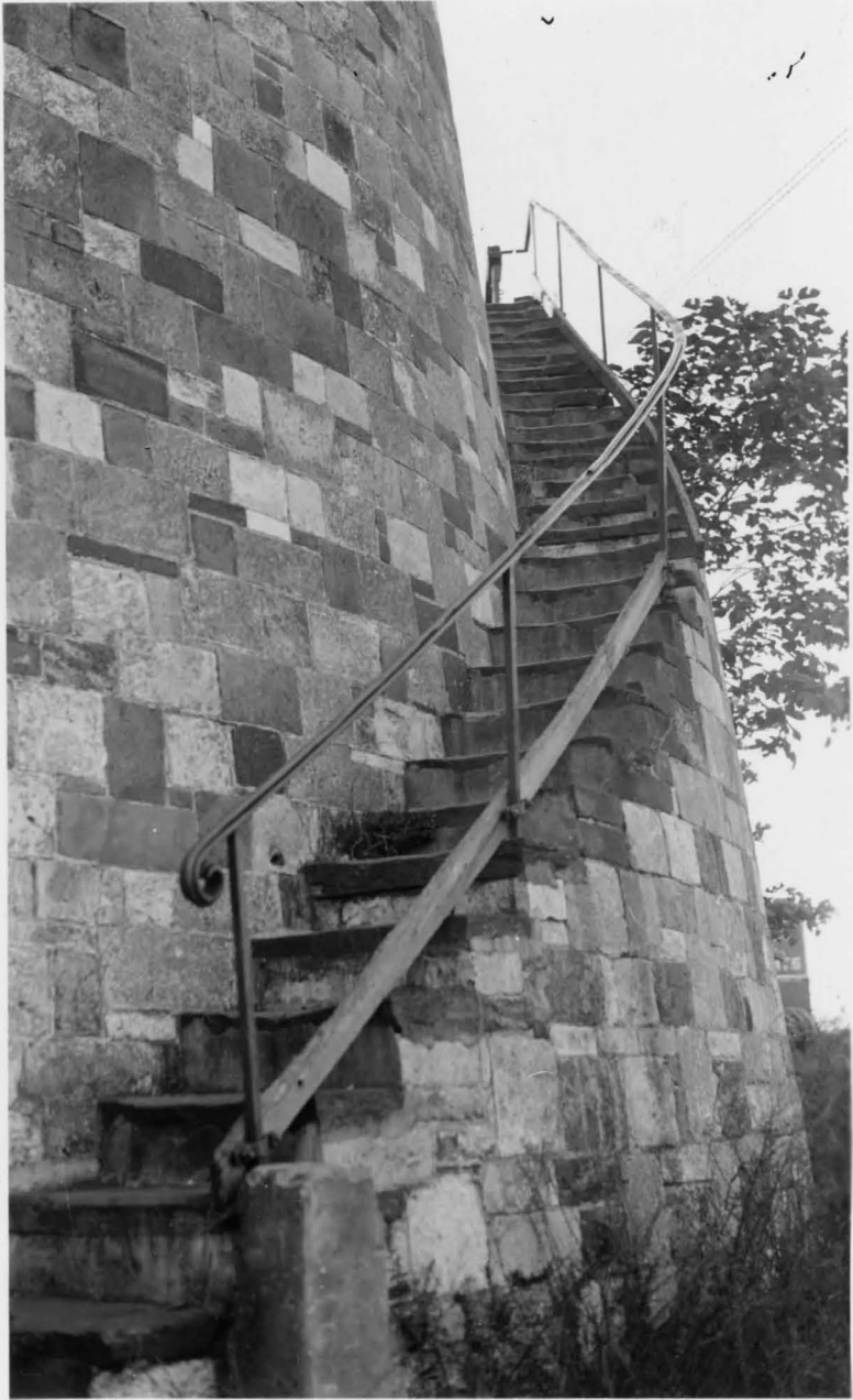
Granite retaining Walls, Savannah River Bluff, with Stair, and Wrought Iron Hand Rail. Foot of East Broad Street.
