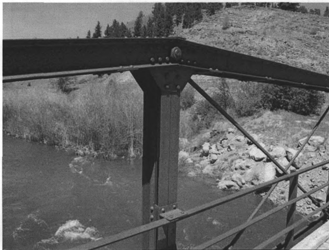
Photograph 0004. Little Blackfoot River Bridge. Detail of upper chord and pin-connection. View to the north.
