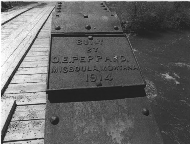
Photograph 0005. Little Blackfoot River Bridge. Detail of dedication plate: "Built by O.E. Peppard. Missoula, Montana. 1914." View to the west.
