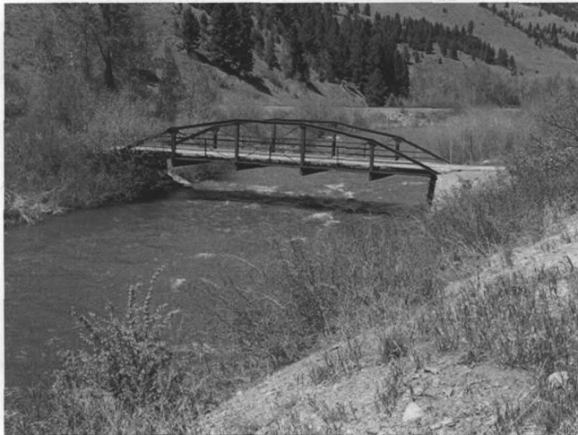
Photograph 0001. Little Blackfoot River Bridge. South profile of truss span. View to the north.
