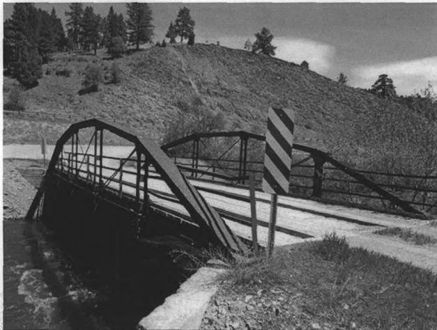
Photograph 0003. Little Blackfoot River Bridge. North profile of truss span and west portal. View to the East-southeast.
