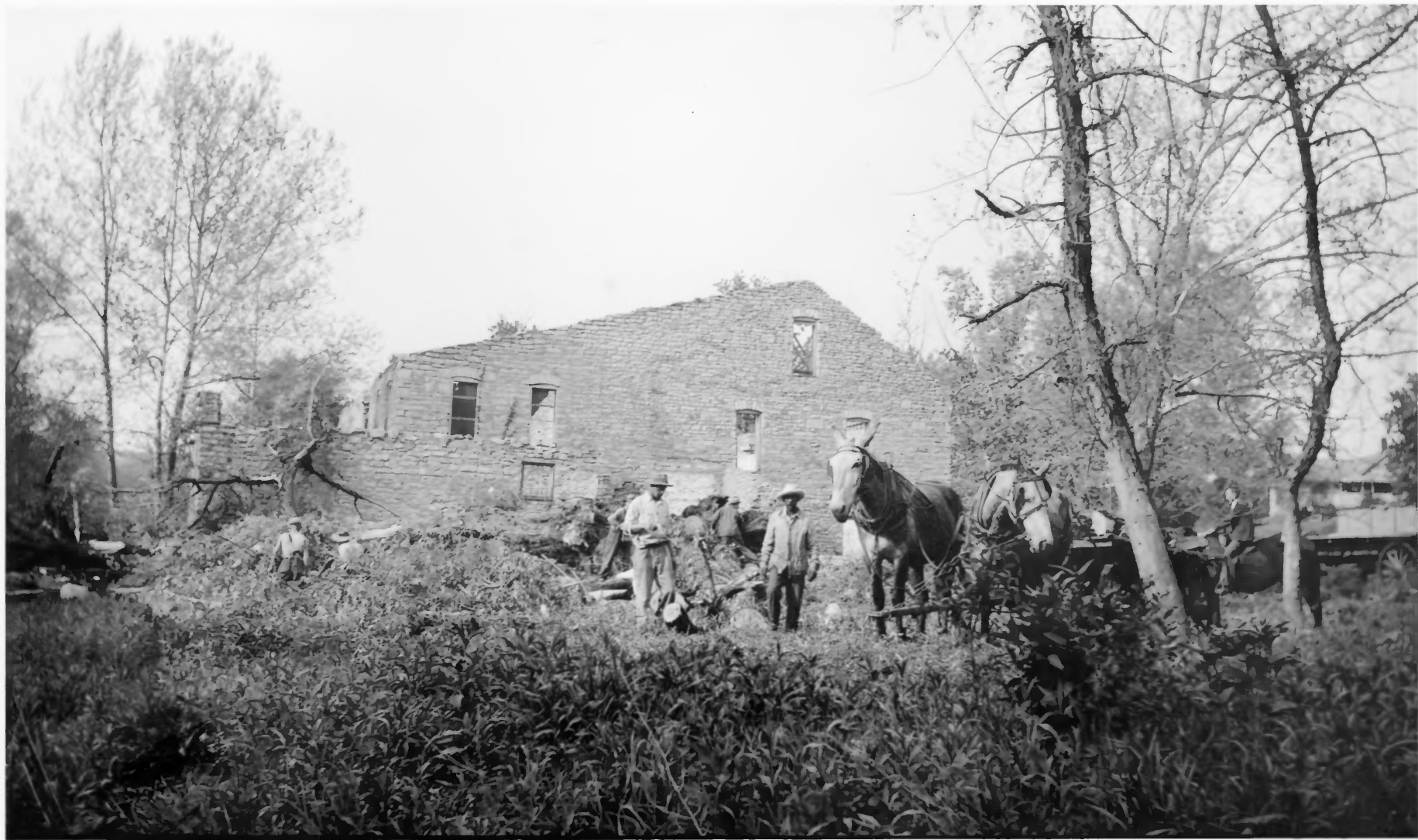
Photo3. LABROT & GRAHAM'S OLD OSCAR PEPPER DISTILLERY Woodford County, Kentucky Clearing underbrush from north side of distillery building Claude V. Bixler, photographer, 1934.
