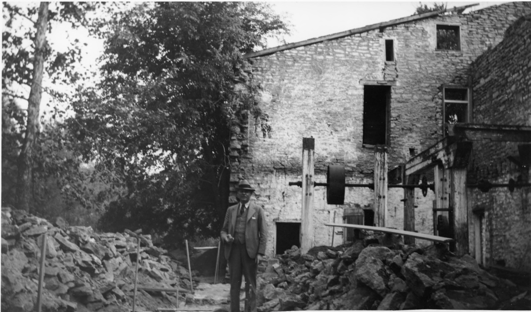
Photo5. LABROT & GRAHAM'S OLD OSCAR PEPPER DISTILLERY Woodford County, Kentucky Distillery building interior, rear part looking south. Rear wall has been taken down and is being rebuilt. Claude V. Bixler, photographer, 1934.
