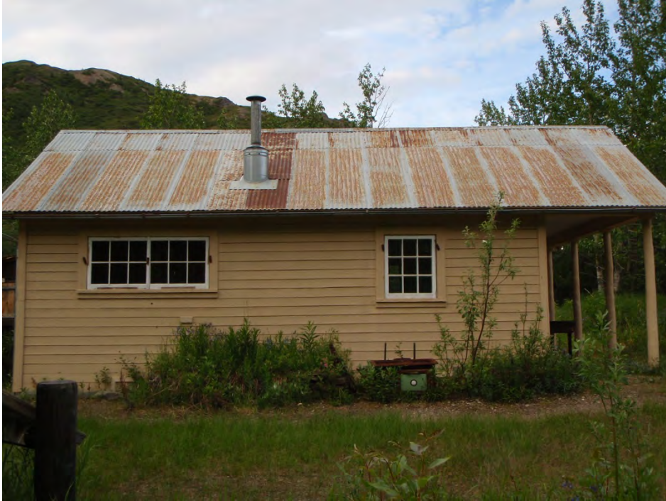
Photo #27 of 29 . (AK_Denali Borough_ Fannie Quigley Residence _0027) West elevation raised planting bed number 2, camera facing northeast.
