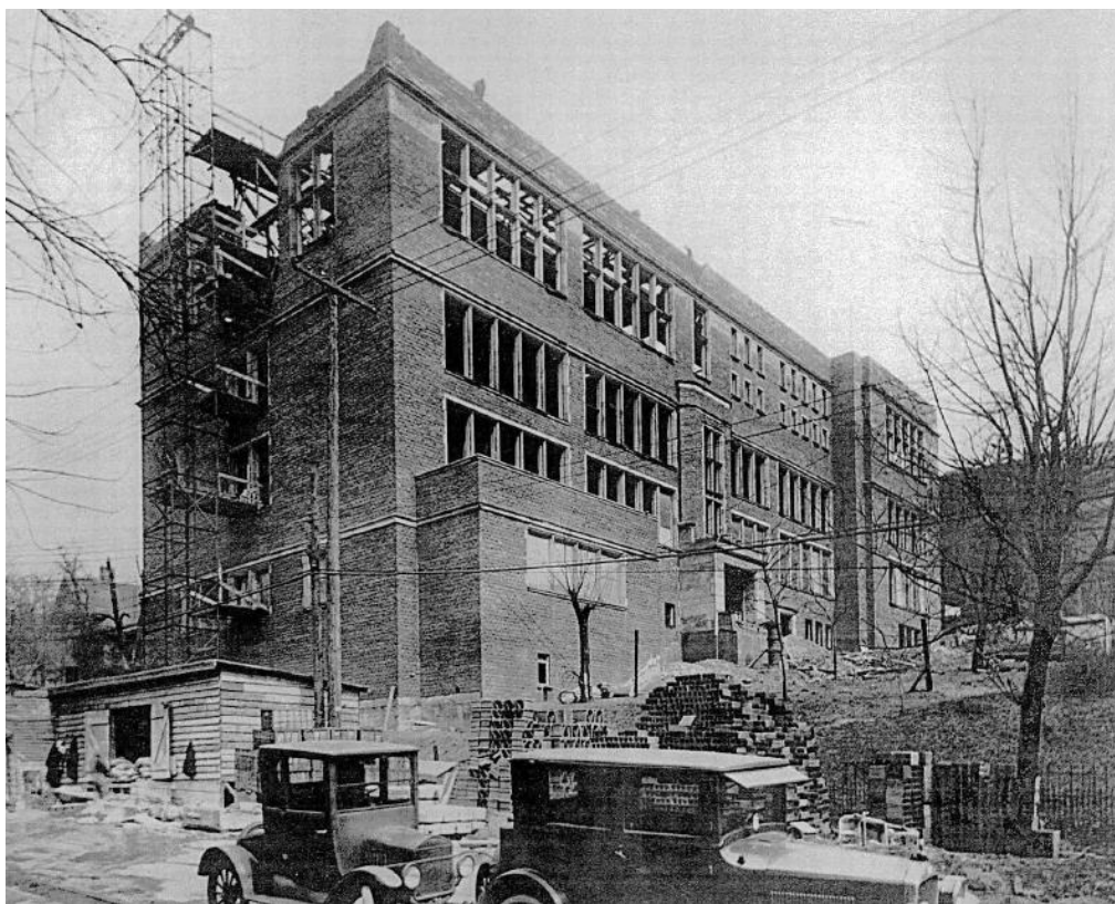
Figure 9: Photograph from March 22, 1926 Showing Construction of the 1926 Annex. Image Source: Gladstone School Historic Resource Survey Form.
