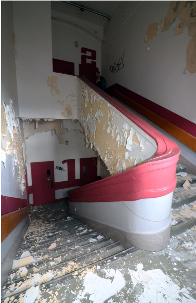
Photo 13: Interior View of a Typical Stairwell, 1914 - 1924 Building, Second Floor, Center West Stairwell, Looking East
