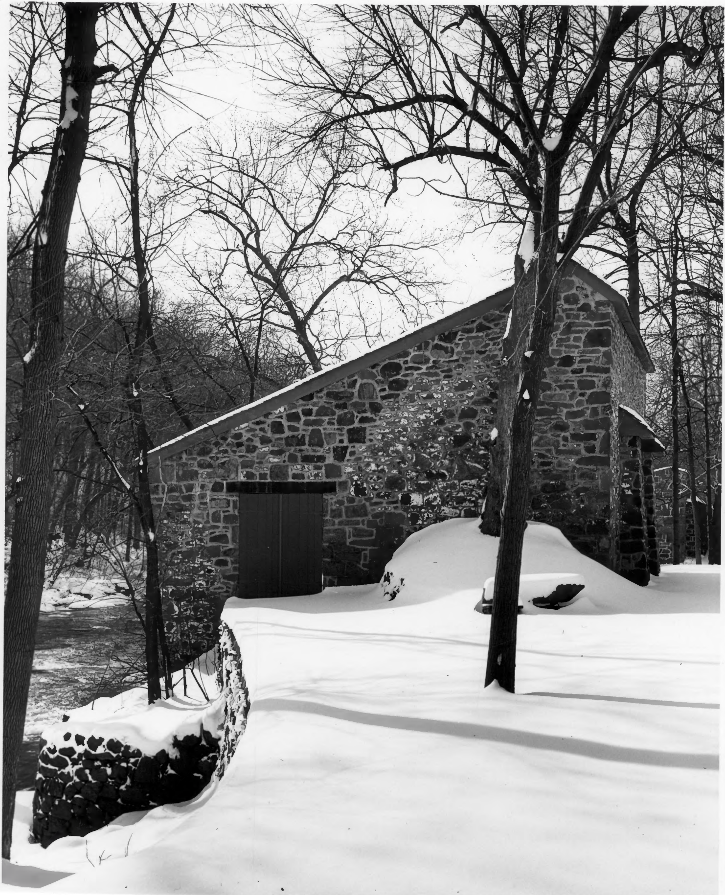
R-13. Glaze Mill - Building shell only. Walls capped in original fashion to prevent deterioration.
