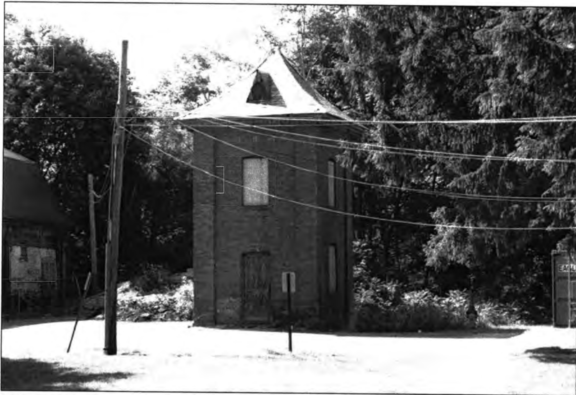
Photo 0012: Exterior view of the Lauralton Hall Water Tower, south and east elevations
