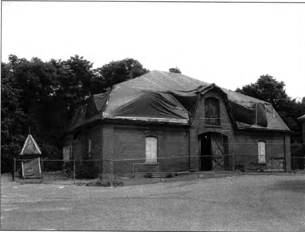
Photo 0009: Exterior view of the Lauralton Hall Carriage House, west and south elevations (Note cupola stored on the ground at left)
