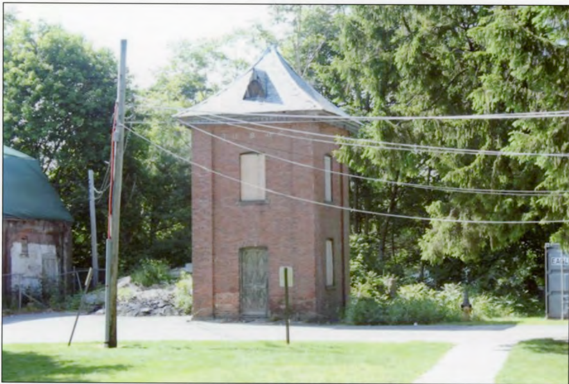
Photo 0012: Exterior view of the Lauralton Hall Water Tower, south and east elevations
