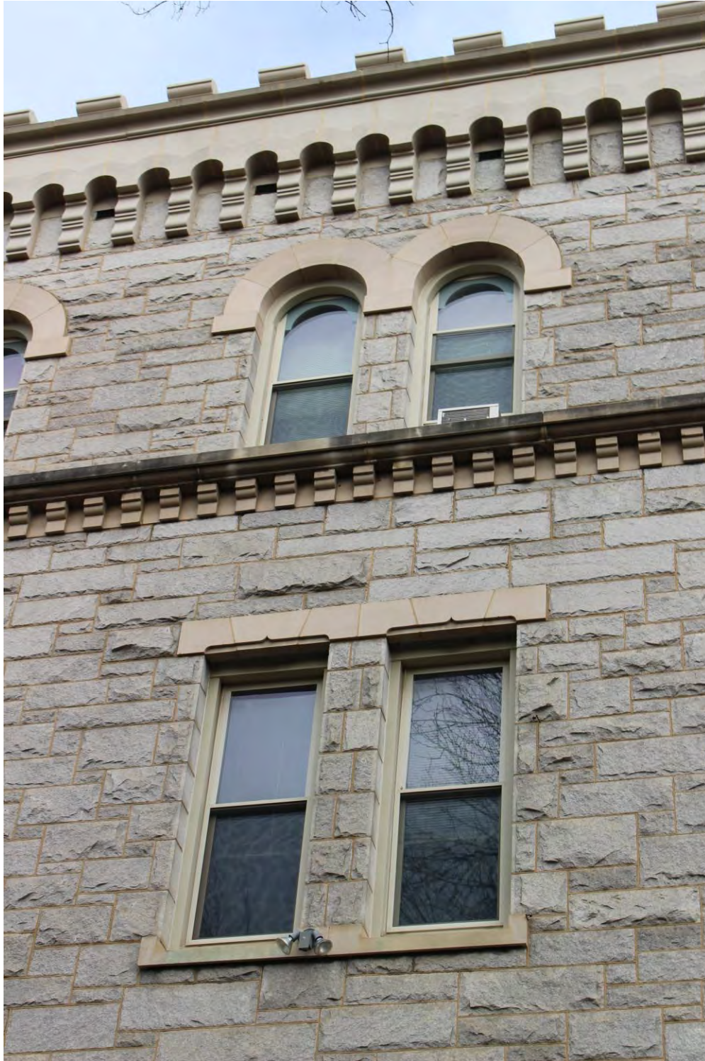
11 of 20 Typical second- and third-story windows and roofline on front elevation, facing west
