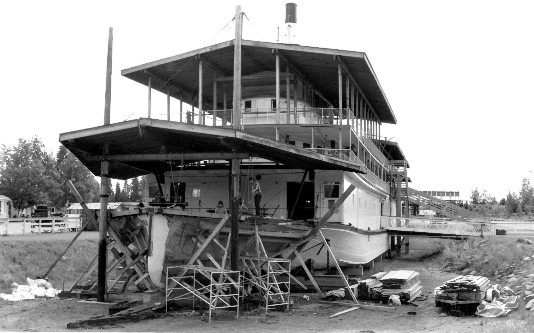
NENANA, Fairbanks, Alaska National Park Service Photograph by William S. Hanable, 1988 City of Fairbanks Port bow quarter view showing restoration work in progress, June 28, 1988. Photo #4
