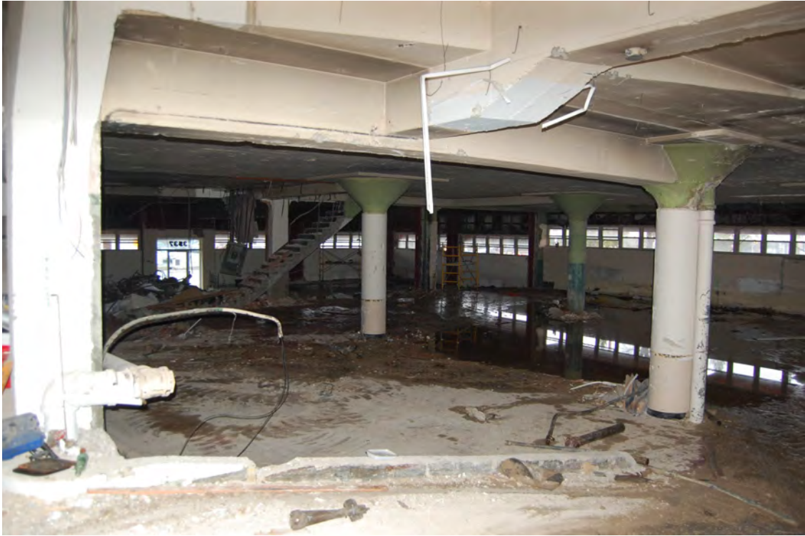
Figure 5. Concrete columns are intact throughout the building. First floor view is southeast.
