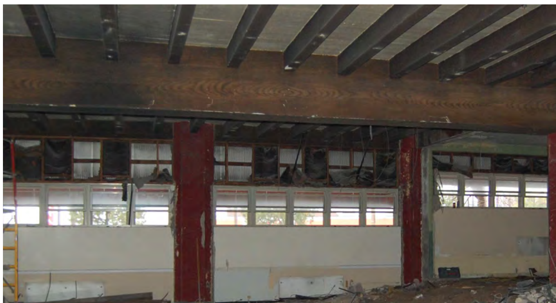
Figure 4. Original clerestory four-light windows above infilled display window bays, first floor, south wall.
