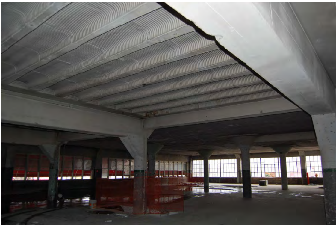
Figure 7. The building is primarily constructed of concrete, including the ceilings. View is second floor, southeast. Note the floor's ribbed concrete ceiling detail.
