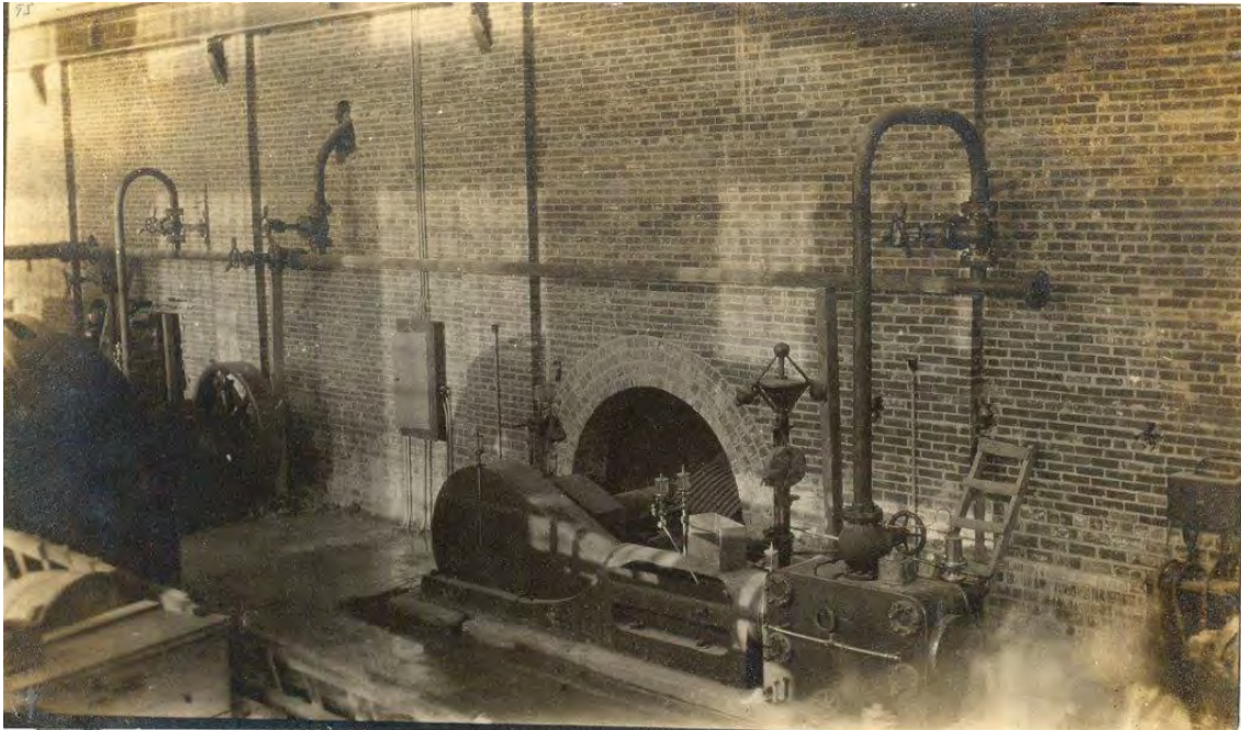
Figure 7. The northeast wall of the southwest 2.5-story power house addition appears much the same as it did in this photo from 1914. Photo courtesy of Robert Abbott.
