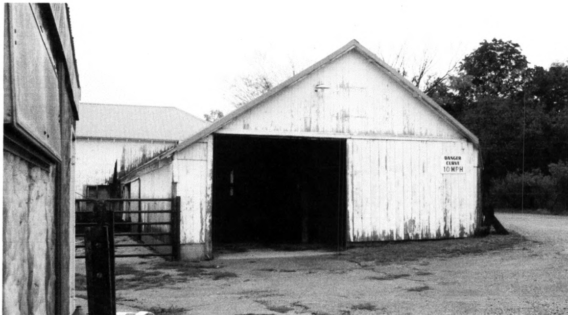
Figure 24 The horse barn (#6) is ell-shaped and pole framed and may date to the 1910-1920 era also. It has exposed rafters. This is the east wing. See Fig. 25 as well. Tallgrass Historians L.C., 2008
