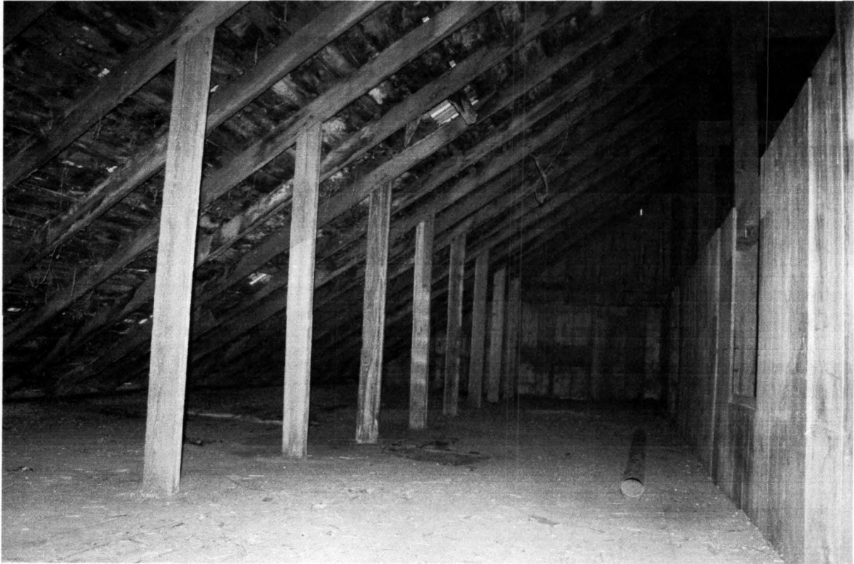
Figure 20 This view of the east side loft bay of the large barn (#3) interior looks south. The plank cross beams of the middle bents and central loft are visible over the partition wall on the right. Tallgrass Historians L.C., 2008
