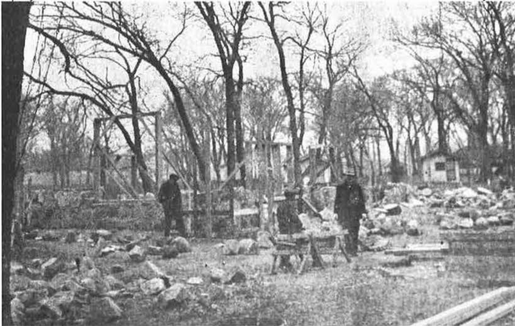
(Image 36) Rocks everywhere to be put in place in the forms erected for the shelter house in Sac City park. Pictured here are Fred Salasek, George Zimmerman, and one of the workers. (Photo Sac Sun , 27 April 1939)
