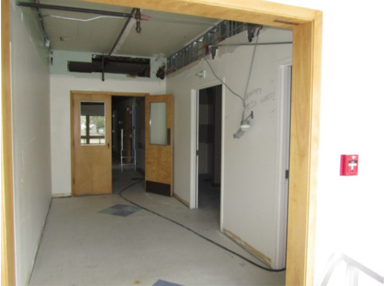
Photo 47: Administrative Corridor, Original Fire Door from Main Entrance Foyer, Aspect: SE
