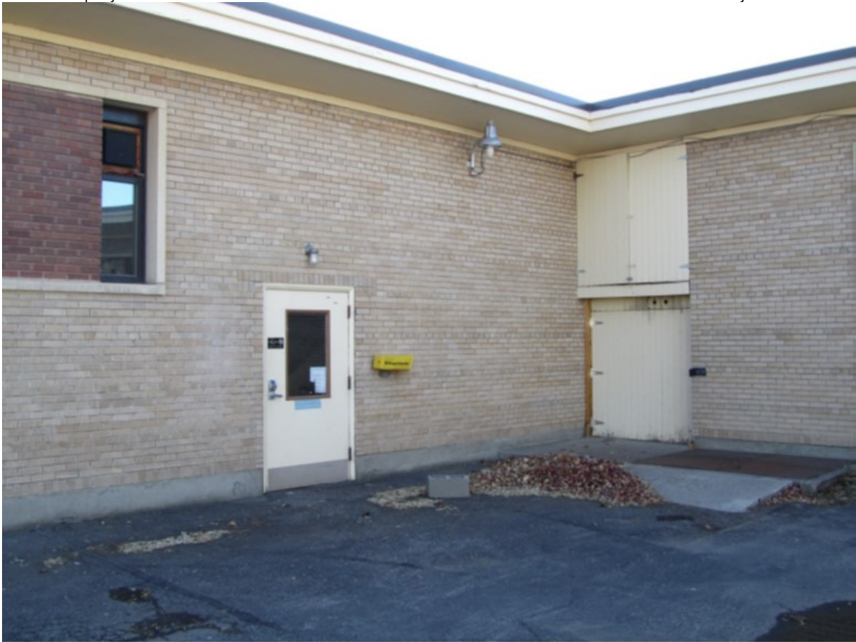
Photo 04. Junction of Hospital Core / Pediatric Wing (NE Elevation) and Administrative Wing (SE Elevation), Aspect: SW
