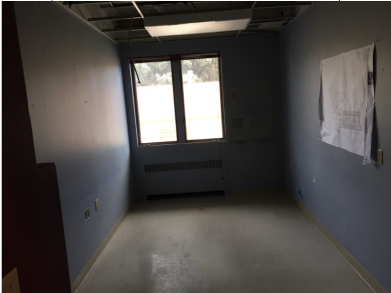
Photo 41: Primary Corridor, Hospital Core (NE side), Typical Room to SE of Administrative Corridor, Aspect: NE
