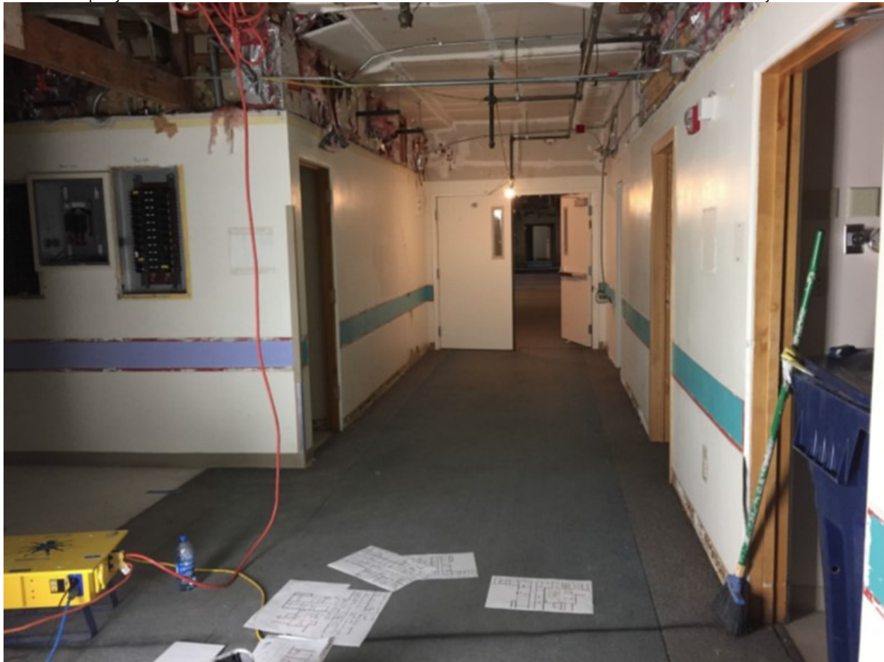
Photo 35: Primary Corridor, Intersection of Hospital Core with Administrative Wing (left), Aspect: SE
