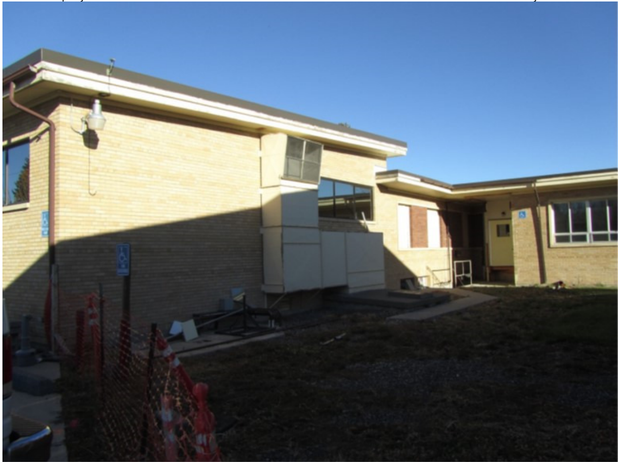
Photo 06. SW Elevation of Surgical Wing with Maternity Wing Hyphen (NW Elevation), Aspect: E
