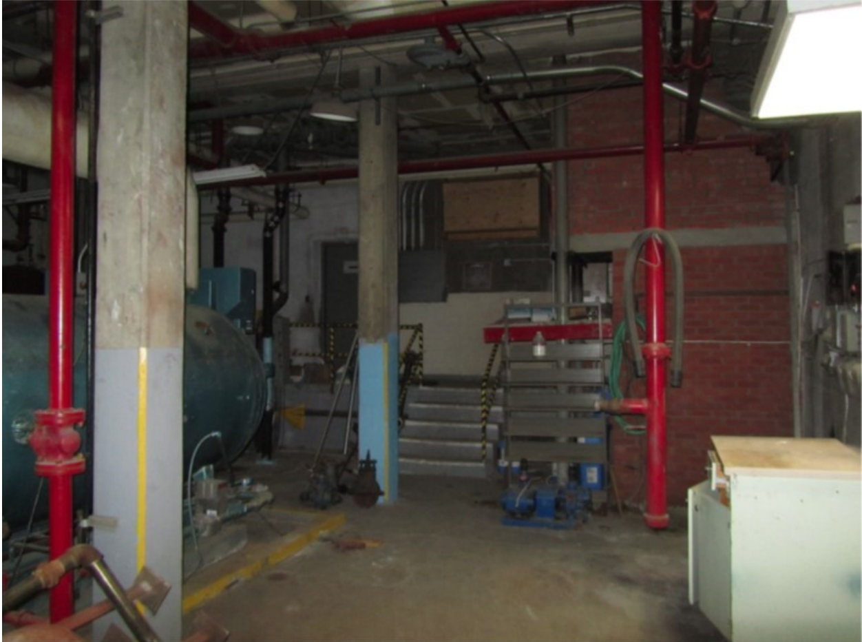
Photo 77: Basement, Administrative Wing, Boiler Room, Aspect: W
