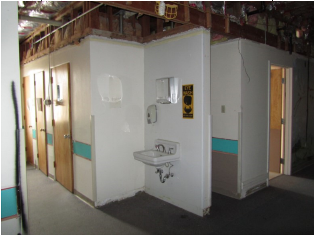
Photo 33: Primary Corridor, Hospital Core, Janitor's Closet and Restrooms (left) and Split-Level Entrance (right), Aspect: E
