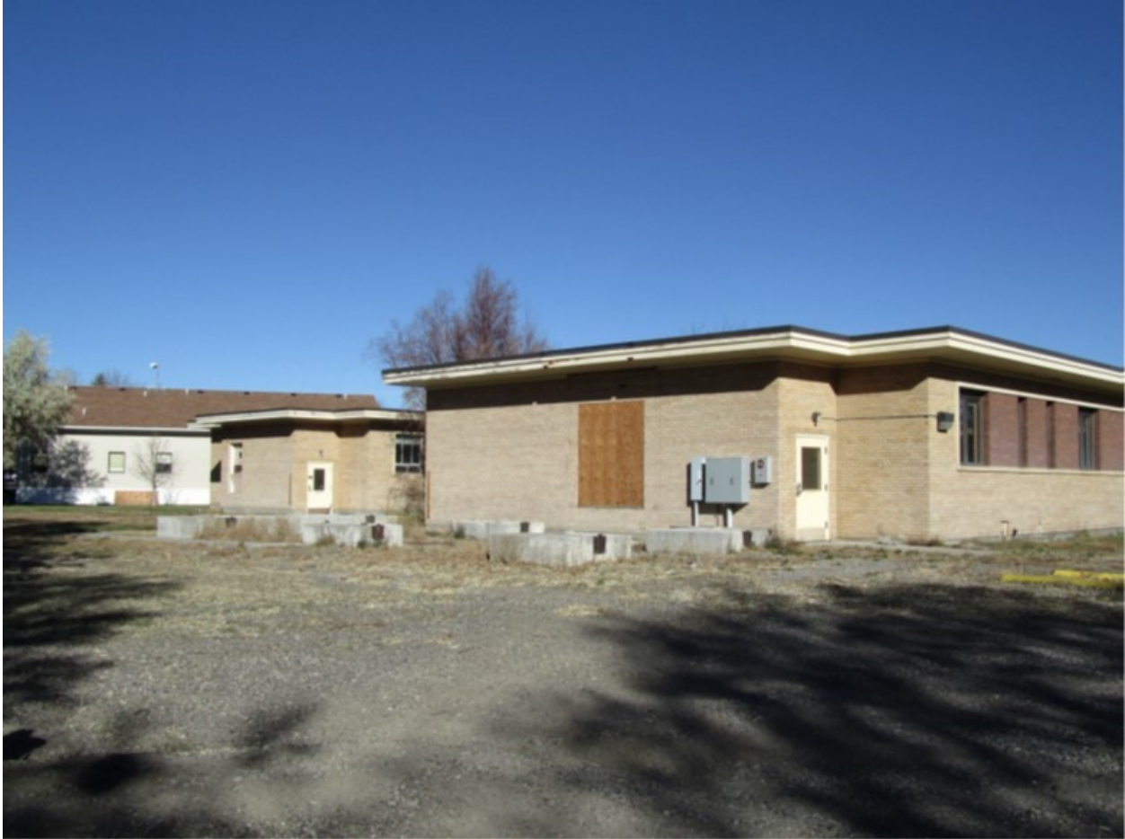
Photo 17: SW Elevation of Nursing Wing (foreground) and SW Elevation of Maternity Wing, Aspect: N
