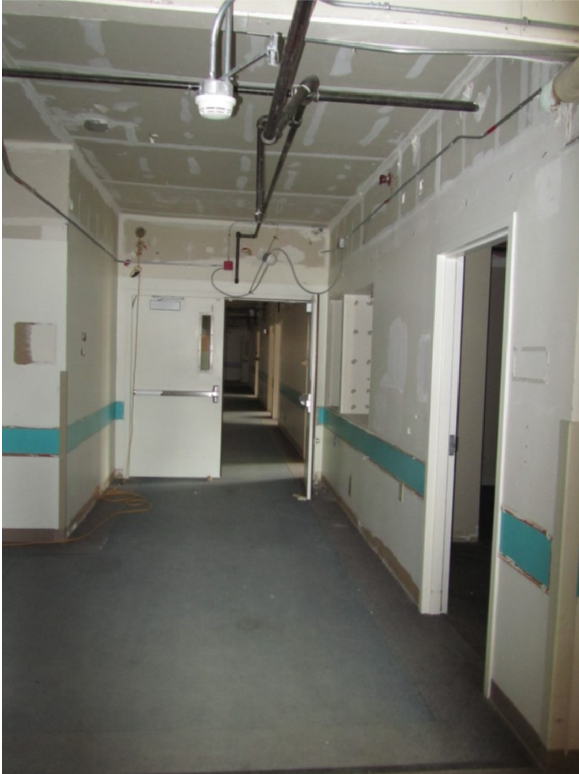
Photo 36: Rooms Addition Corridor, Intersection with Nursing Corridor and Primary Corridor, Aspect: SE
