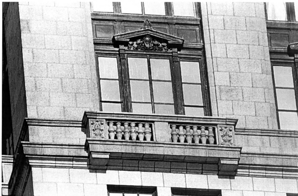
HV-14: Detail view of typical balcony balustrade and pedimented windows at Nineteenth Floor, c. 1990. Courtesy of the Baltimore Gas and Electric Company Archives, Baltimore, Maryland.
