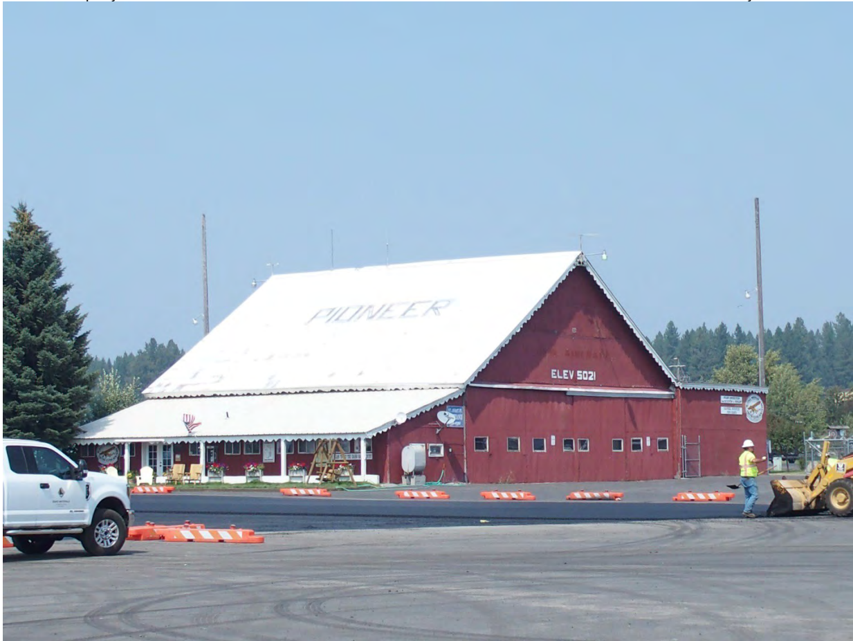
Photo #4 (ID_Valley County_Johnson Flying Service Hangar_0004) Façade, southwest elevation and southeast elevation, camera facing north.
