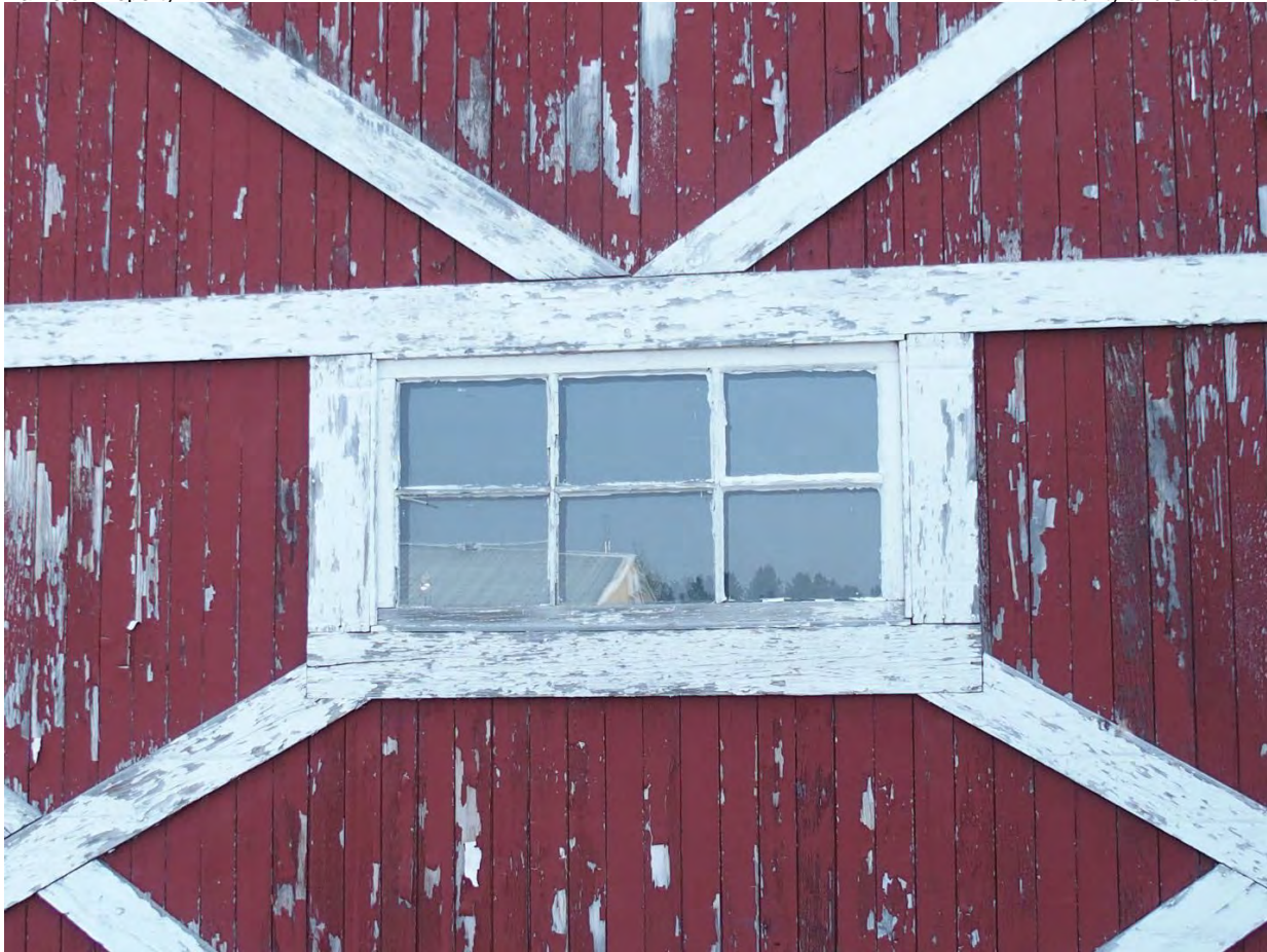
Photo #10: (ID_Valley County_Johnson Flying Service Hangar_0010) Northwest elevation. Window detail,,camera facing south.
