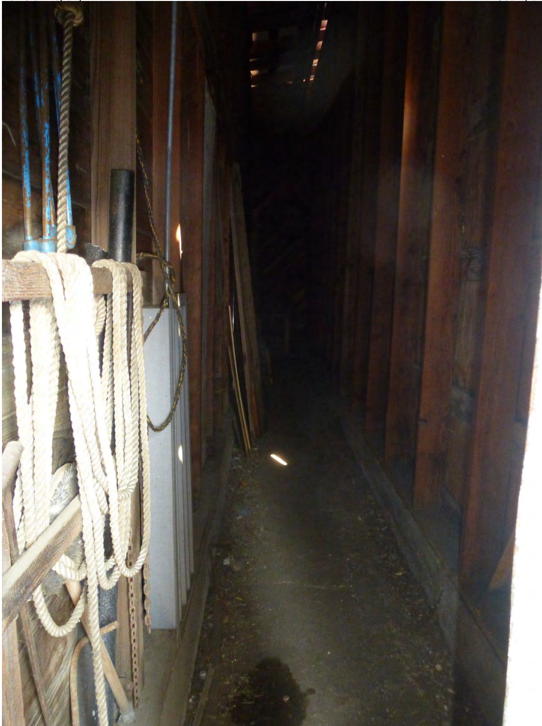
Photo # 16 (ID_Valley County_Johnson Flying Service Hangar_0016) Interior view hangar door storage compartment,,camera facing east.
