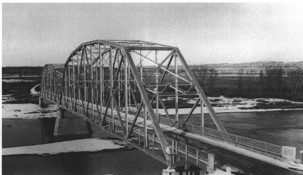
Photograph 0001. Big Horn River Bridge. North profile and west portal. View to the southeast.
