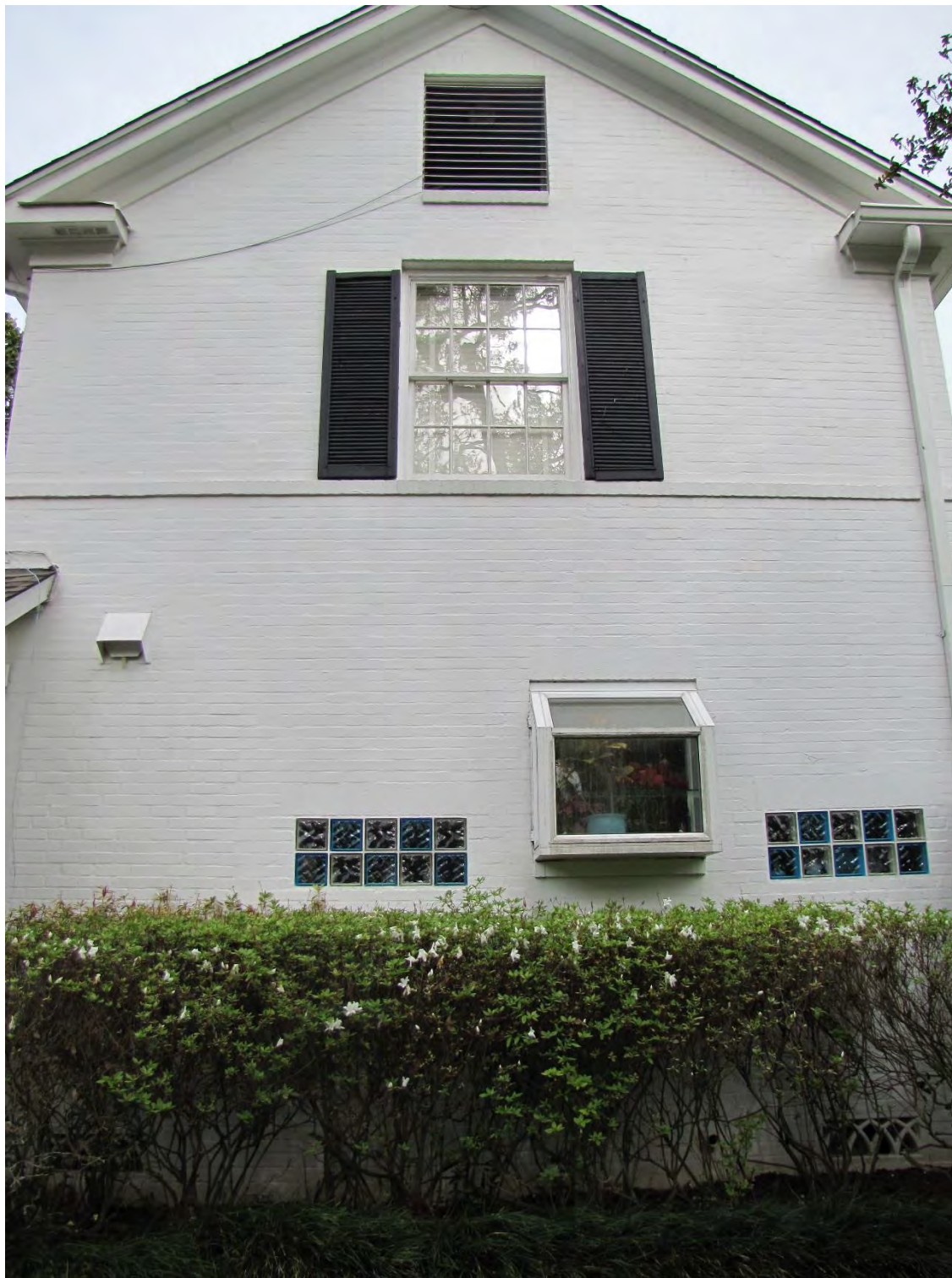
Photo 7: West elevation. Projecting garden bay and prism glass windows visible. Camera facing east.
