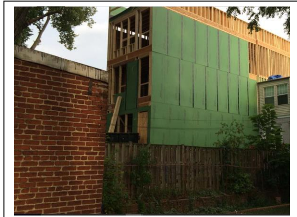
POP-up while still being constructed @ 67 V street NW, adjacent to my home at 69 V street (the small house on the right)
