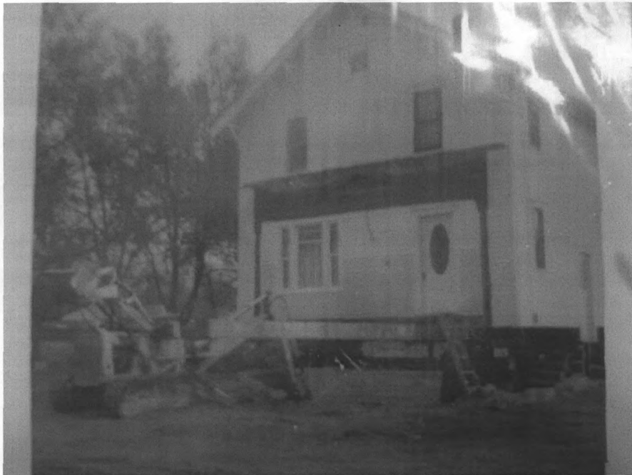
New foundation installed and front porch removed, 1972. The Nunbergs completed the front addition in 1974.
