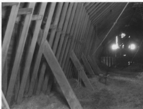
Figure 3 The loft floor of the barn on Tyden Farm No. 6 is virtually unencumbered by structural framing because of the sidewall truss system that forms the roof. (Tallgrass Historians L.C., 2007)
