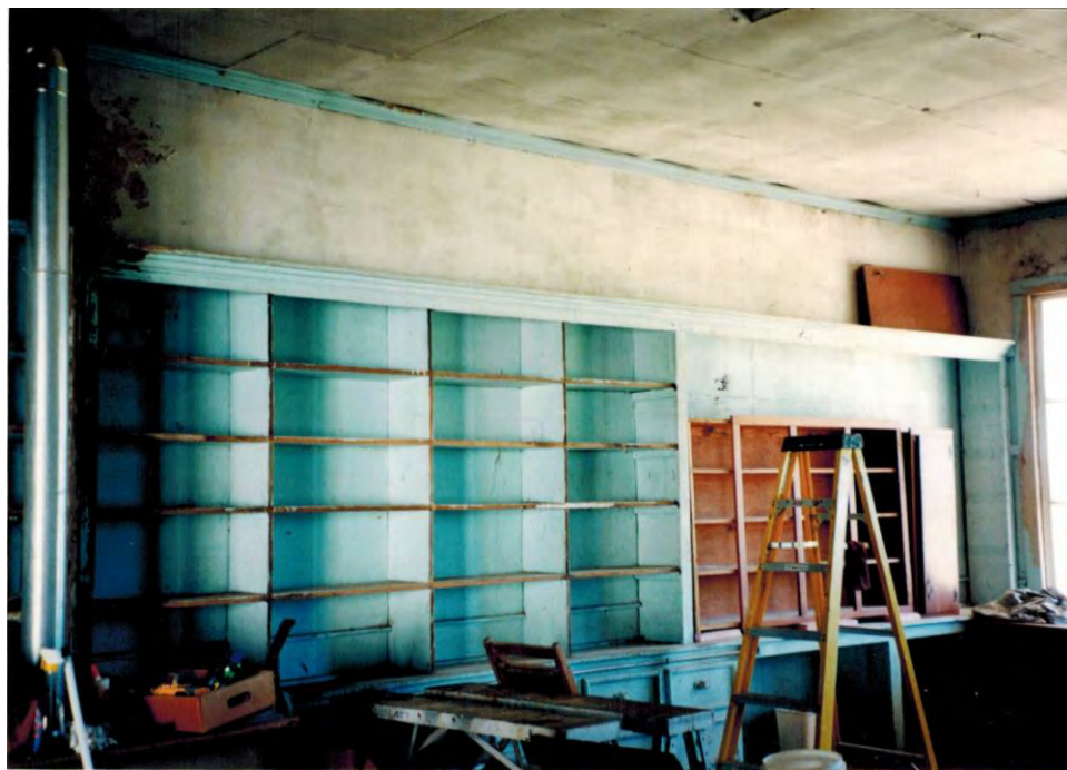
Figure 12. Store, interior view of east wall and doors, and east end of south wall, camera facing southeast
