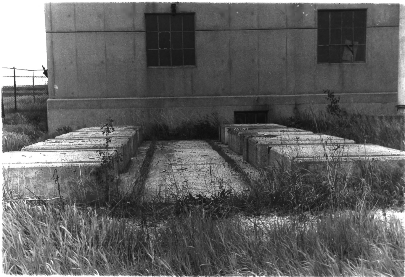
REA PLANT - Franklin Co., Iowa - Item VI - Photo G Location of transformers.
