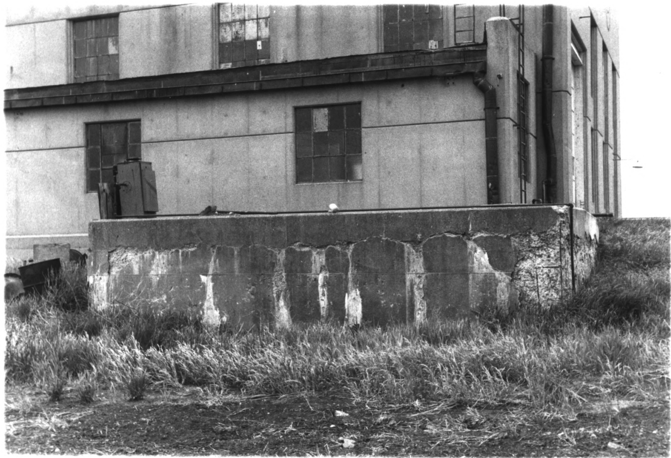
REA PLANT - Franklin Co., Iowa - Item VI Photo E Sump tank
