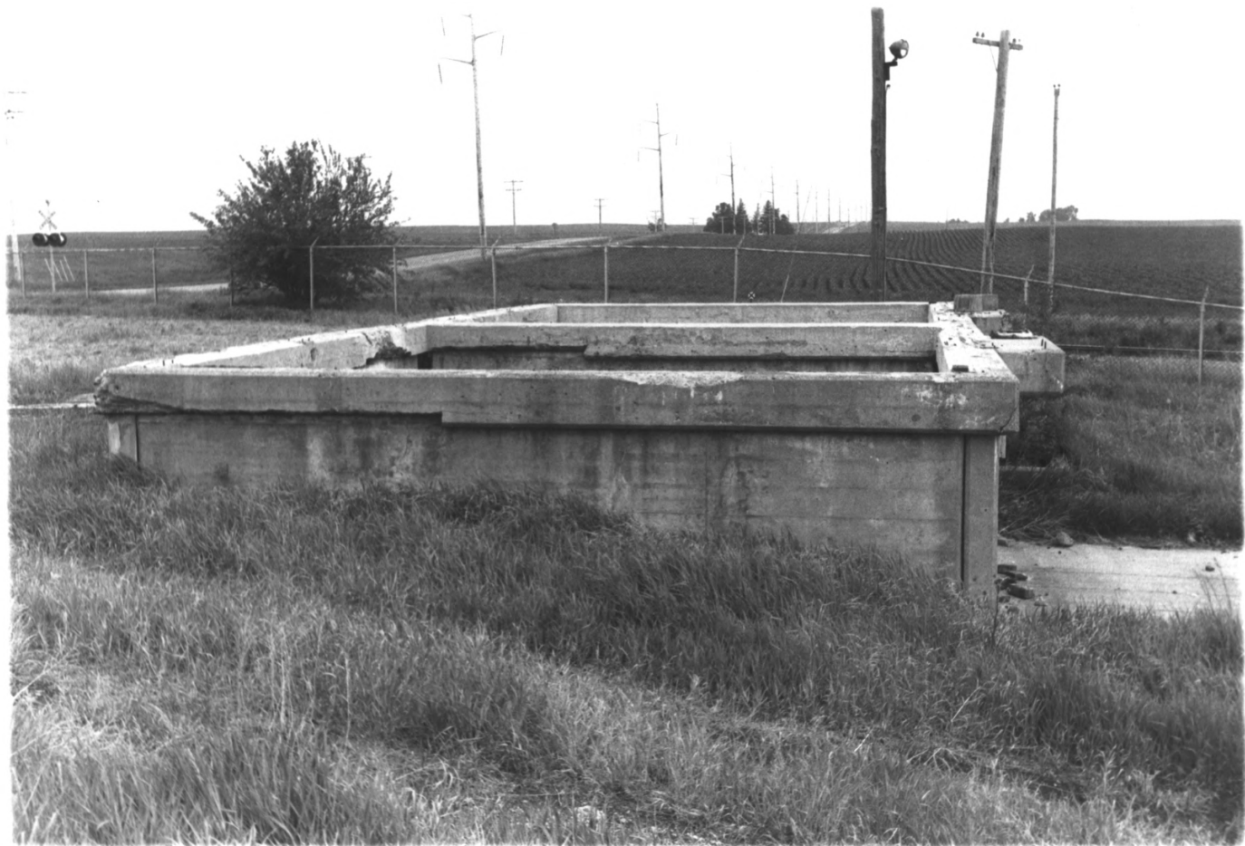
REA PLANT - Franklin Co., Iowa - Item VI (Photo D) Water cooling tanks (towers).
